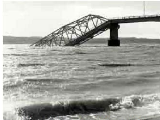
Hood Canal Bridge – February 13, 1979 (WSDOT)
