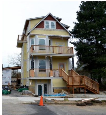
Right image: An old Victorian house in Portland being internally divided into a fourplex. Source: Michael Anderson.
