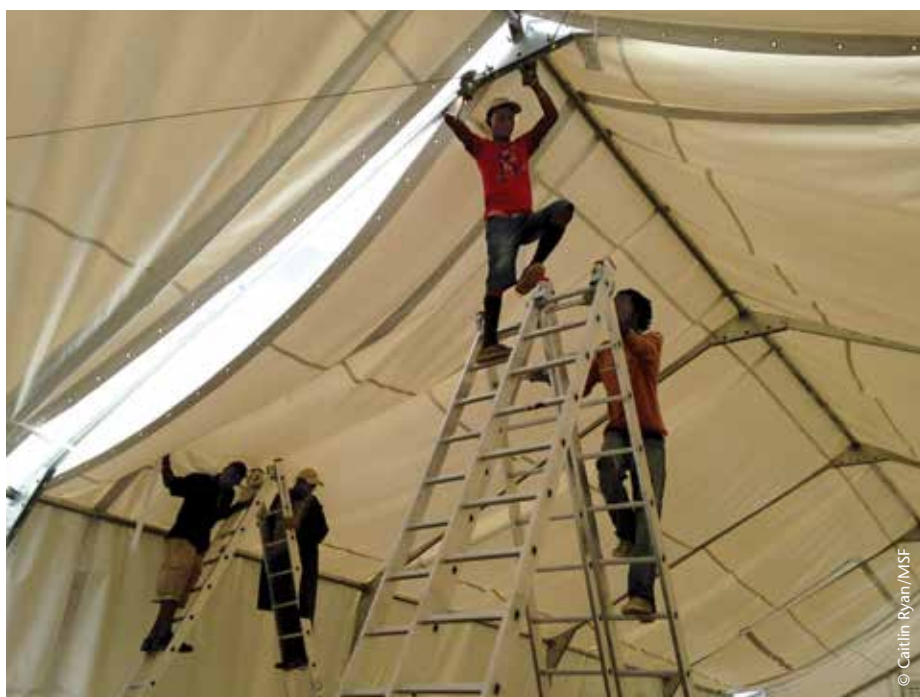
Construction teams building what will become one of the wards at ELWA 3, MSF's EMC on the outskirts of Monrovia.
