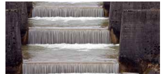
Particularly in whitewater, concrete surfaces are subject to massive additional strains by rubble, sharp edges and abrasion, as well as possible temperature stresses due to frost exposure.
