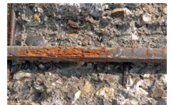
Damage to concrete structure due to insufficient concrete cover and low concrete quality
