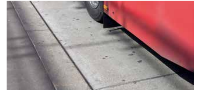
Concrete roadways and other publicly accessible areas, especially those experiencing high volumes of traffic or concentrated loads, are subject alongside high mechanical burdens also to strong abrasion, often presenting the risk of a smooth, slick surface.
