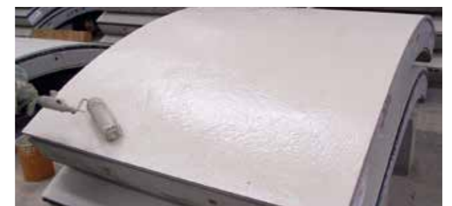
Immediately following curing in a steam channel, the concrete surface of tunnel lining segments is coated with water-based epoxy emulsion that is absorbed even into the smallest pores, thereby generating a sealed, protective coating.
