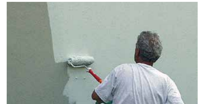
Epoxy resin-based protective coatings are applied over the entire surface following reprofiling of the concrete surface with sulfate-resistant repair mortar enhanced with synthetic material.
