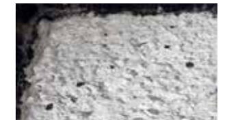
Very severe surface weathering
