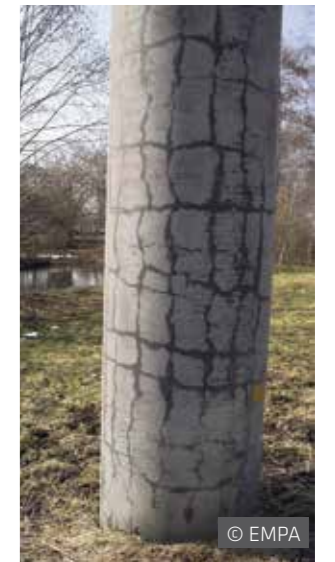
The appearance of ASR damage can be assessed very well on the drying concrete surface of this bridge pylon. Damage can appear within years or only after decades.
