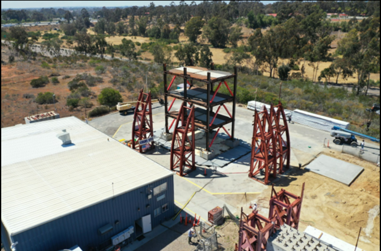
Figure 1. Modular test bed building fully assembled at LHPOST6 prior to shake table testing: special moment frames in the longitudinal direction, buckling restrained brace frames in the transverse direction.
