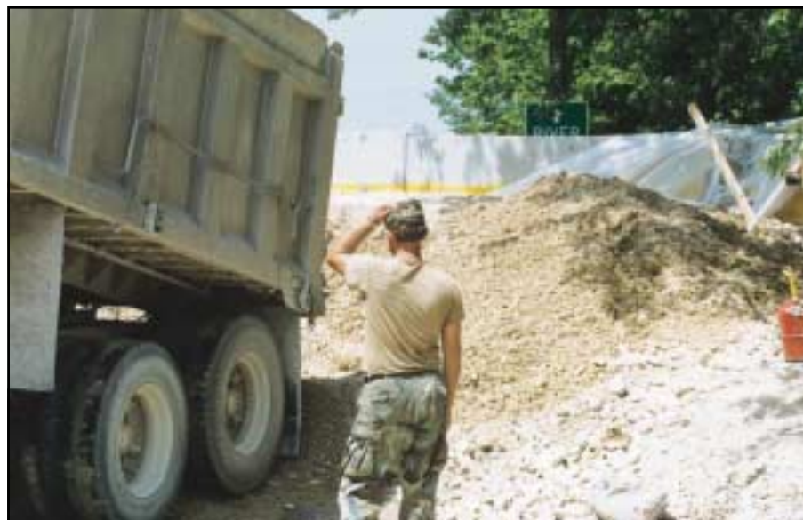
The Missouri Army National Guard reinforced parts of the levee at Ste. Genevieve with 400,000 tons of rock and mine tailings.
