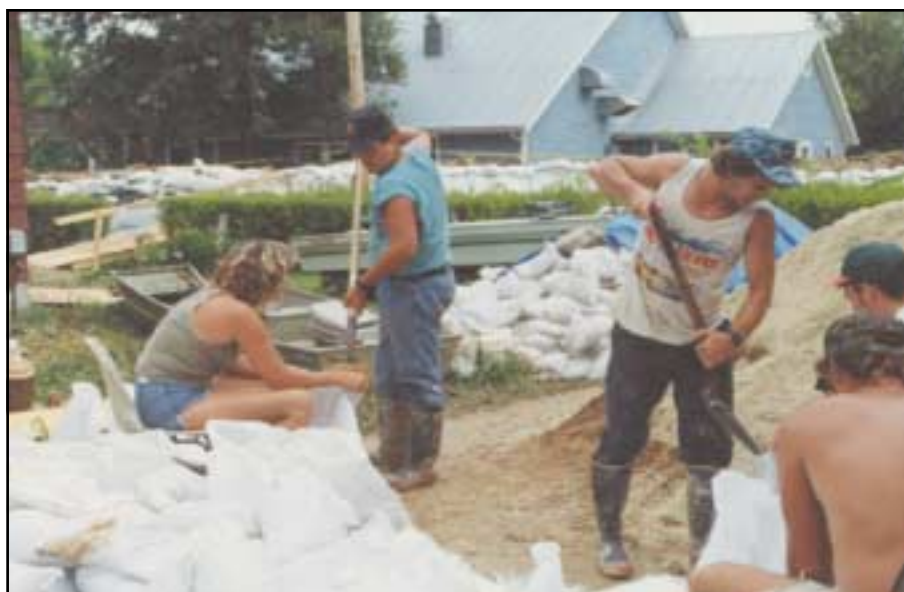
Volunteers work to erect a sandbag levee in the St. Louis area.
