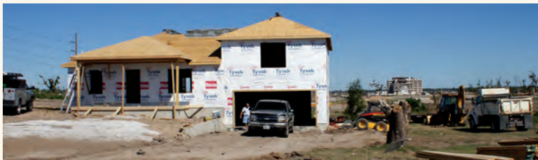
Sept. 8: With the destroyed hospital in the distance, a home takes shape.
