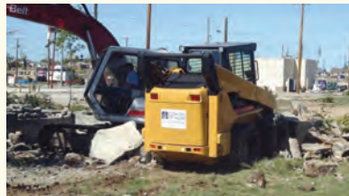
Convoy of Hope demolishes home foundations. Faith-based organizations cleared debris and demolished destroyed homes.
