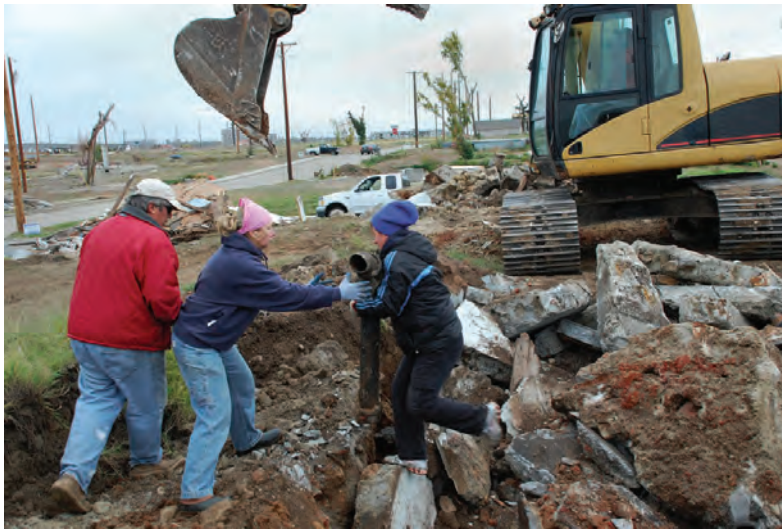
Left: United Methodist Church volunteers demolish and clear a concrete slab for an uninsured homeowner. Below: Springfield-based Convoy of Hope, less than 75 miles from Joplin, was rapidly lending a hand.
