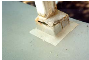
RAIL POST DEGRADATION
