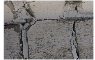
SEALANT ADHESION FAILURE
