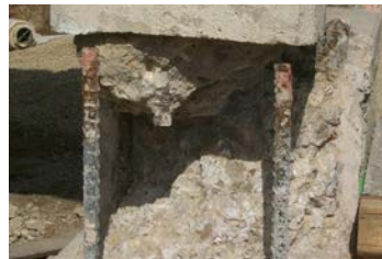
POOR CONCRETE COVER
