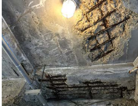
Exposed steel due to corrosion
