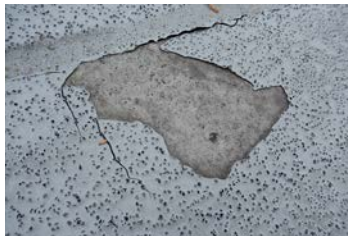
FAILED DECK COATINGS
