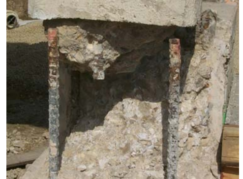
Severely damaged concrete columns accelerated by lack of adequate cover
