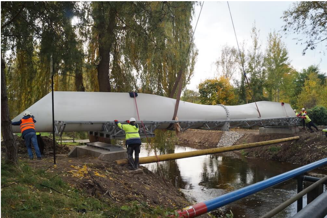
Figure 1. Construction workers install a footbridge across the Szprotawa River in Poland. The footbridge was designed and constructed by Anmet, a Polish recycling company, whose designs feature repurposed wind turbine blades. Photo from Anmet.
