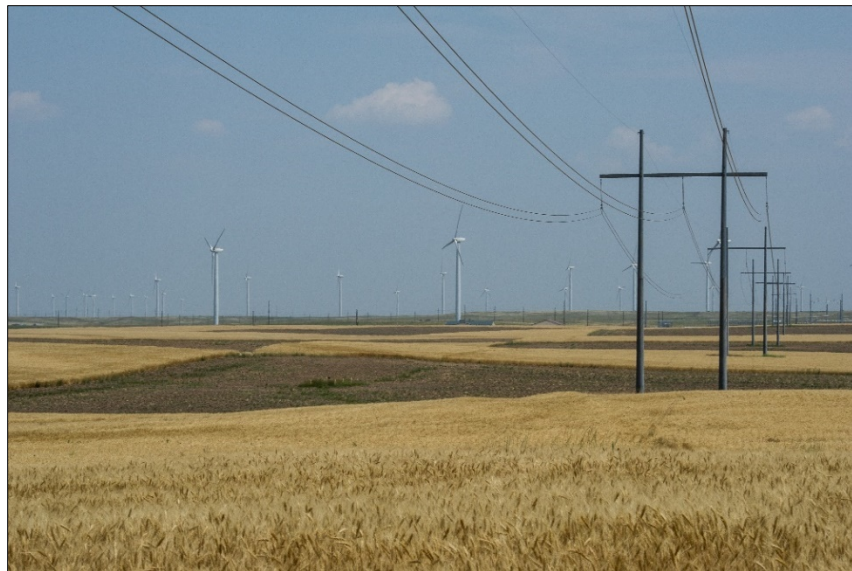
Figure 10. Utility-scale wind turbines and transmission lines at the Cedar Creek Wind Farm in Grover, Colorado. Photo by Dennis Schroeder, NREL 31198
