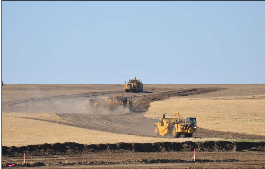
Figure 17. The construction of access roads for the Tucannon River Wind Farm near Dayton, Washington. Photo from Portland General Electric
