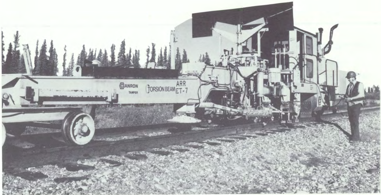
The Railroad completed one of its largest major maintenance-of-way programs. This torsion beam tie tamper does the work of 52 men per day.
