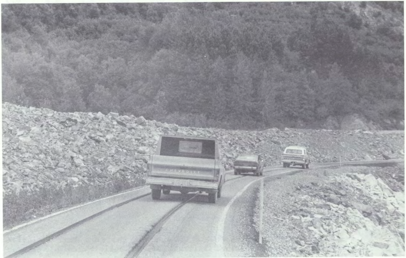
Railbed paving keeps vehicles moving around a major highway reconstruction project on the Seward Highway.
