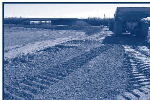
Railroad land on the west end of the Fairbanks Rail Yard and just west of the Johansen Expressway overpass is being filled and leveled as part of a fuel terminal development.
