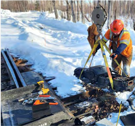
In 2022, construction got underway to replace aging powered switch machines from Portage to Hurricane. The machines allow a switch to be controlled remotely.
