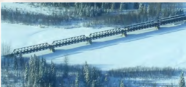
Work began in 2018 to replace the multi-span bridge at MP 147.5, which spans the North Channel of the Knik River.
