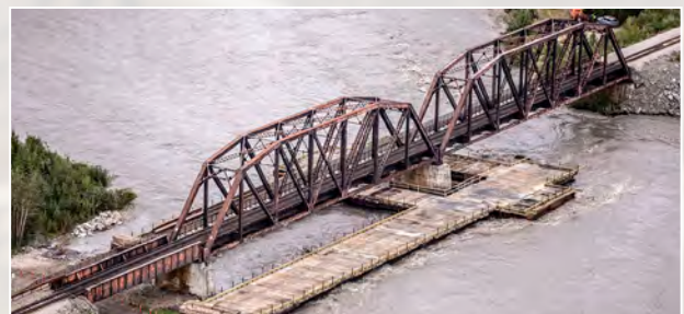
Construction began to replace the center pier on the bridge over the Nenana River at MP 370.7. Bridge infrastructure was compromised during the floods of 2012.
