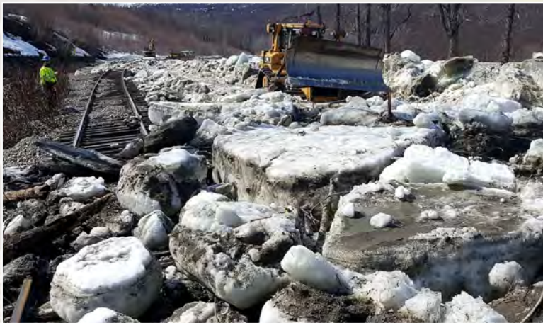
Heavy equipment moves massive ice chunks from the rail corridor as the railroad responds to late spring flooding and ice flows along the Susitna River.
