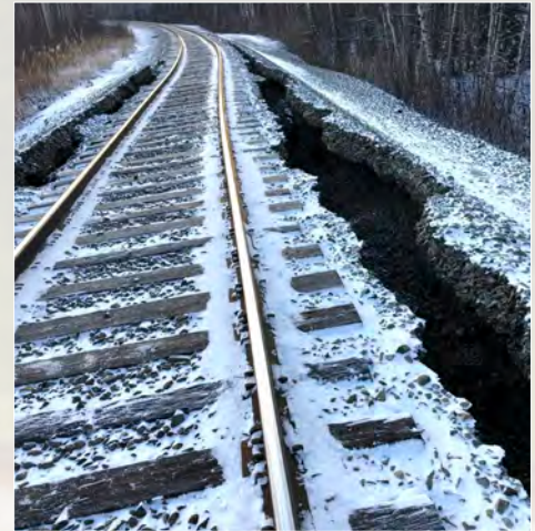
A 7.1 magnitude earthquake split sections of the trackbed during severe shaking Nov. 30.
