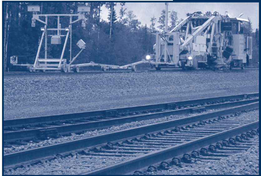
Surfacing on a segment of the Port MacKenzie Rail Extension project, which is slated to be complete by 2017.
