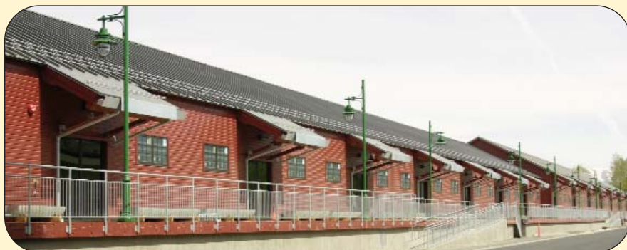
RENOVATING THE HISTORIC FREIGHT SHED TO LEADERSHIP ENERGY & ENVIRONMENTAL DESIGN (LEED) STANDARDS IS A MAJOR INTERNALLY-FUNDED PROJECT.
