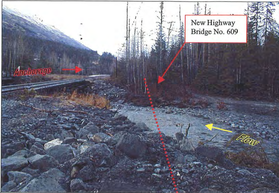
Looking north along new highway bridge alignment. Cobbles and boulders in foreground are for existing railroad embankment.
