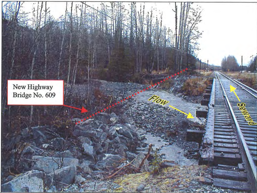
Looking south along highway Bridge No. 609 alignment. Cobbles and boulders present along this alignment.
