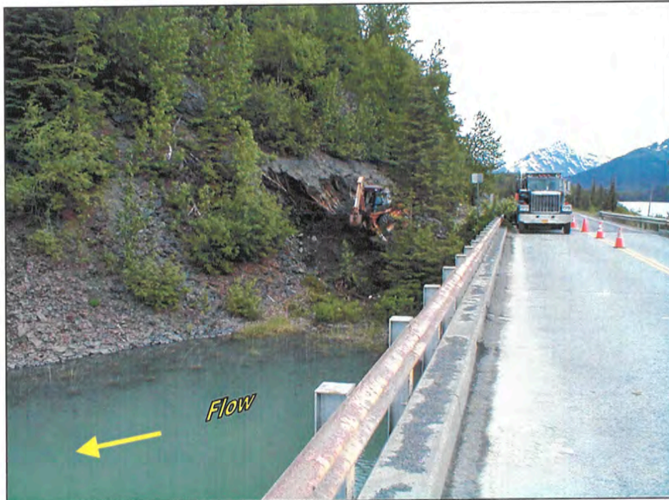
Looking at the proposed location of Abutment No. 5 from center of the existing bridge. The excavator is at the location of Test Pit 13.
