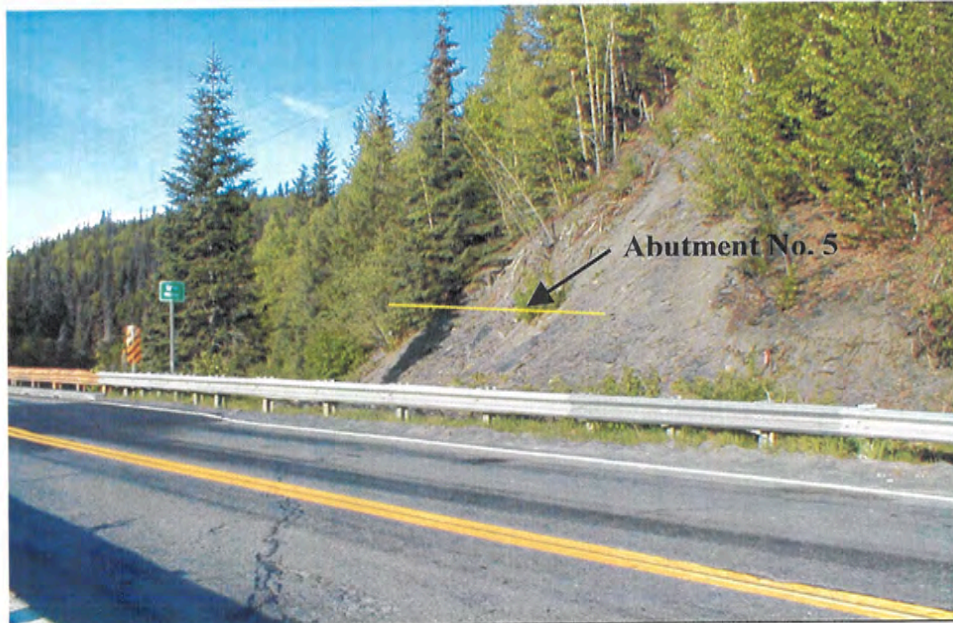
View of proposed Abutment 5. Note the very steep hillside debris and bedrock slope.
