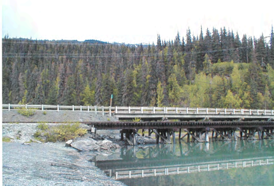
Looking west at the existing southern abutment of the highway and AKRR bridges. Only about 6 m separates the two bridges.
