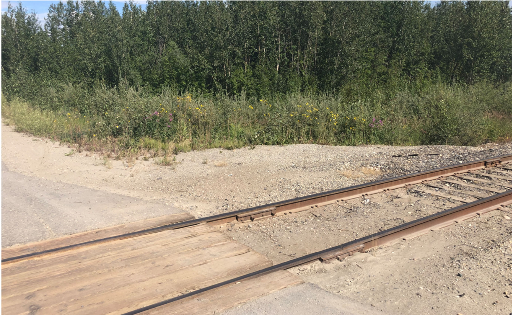
Figure 5 - Joints on East Side (July 2021)
