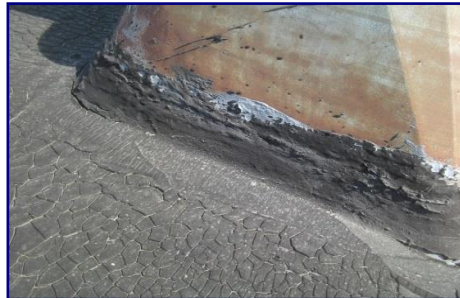
Roof Vent Mastic
