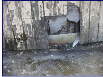
Damage Roof wall
