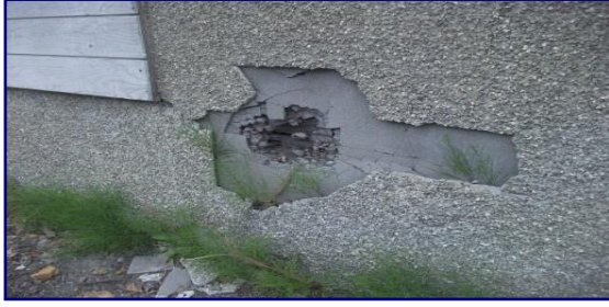
Front Lathe and Plaster Wall
