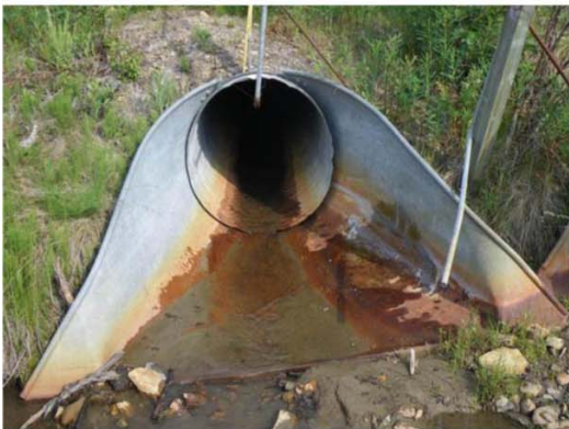
Flared Metal Apron Culvert
