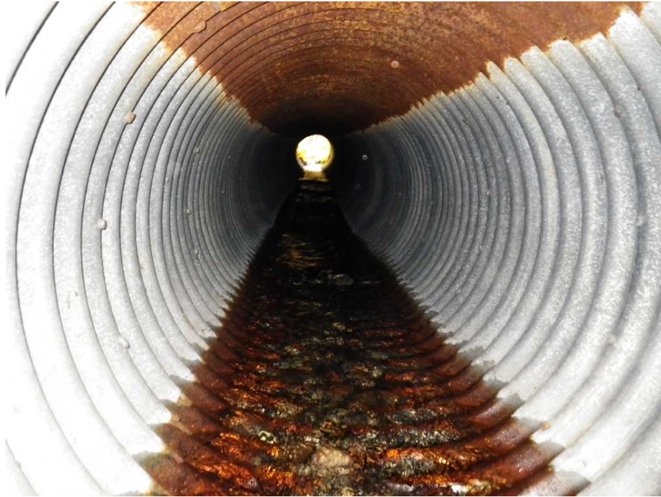
Figure 14b. Culvert showing multiple rust lines due to reuse.
