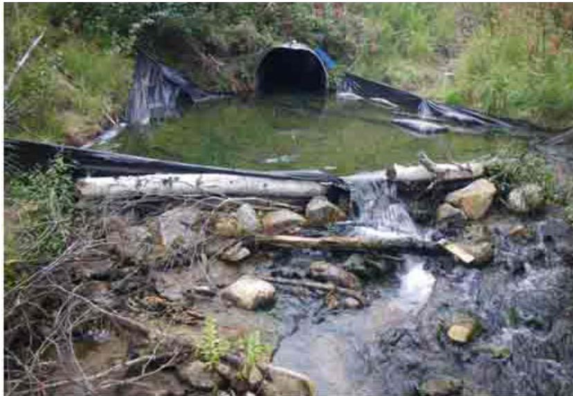
Figure 40c.–Photograph of a passage barrier downstream of culvert.
