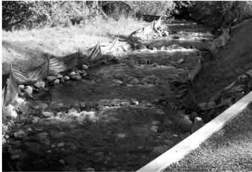
Figure 25a.—Looking upstream at a series of step pools constructed as part of a replacement project.
