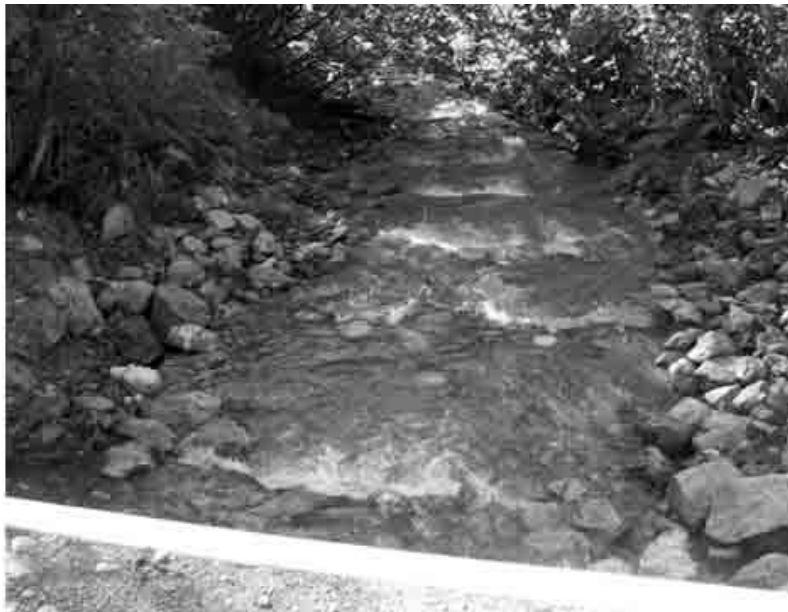
Figure 25b.—Looking downstream at a series of step pools constructed as part of a culvert replacement project.
