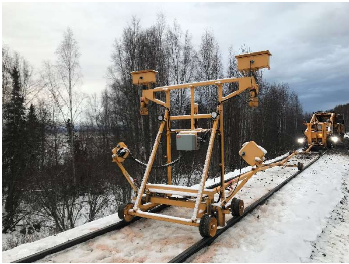
Photo 3: The ET20 realigning and raising the rail at ≈MP138.5, looking RR North-Northwest.
