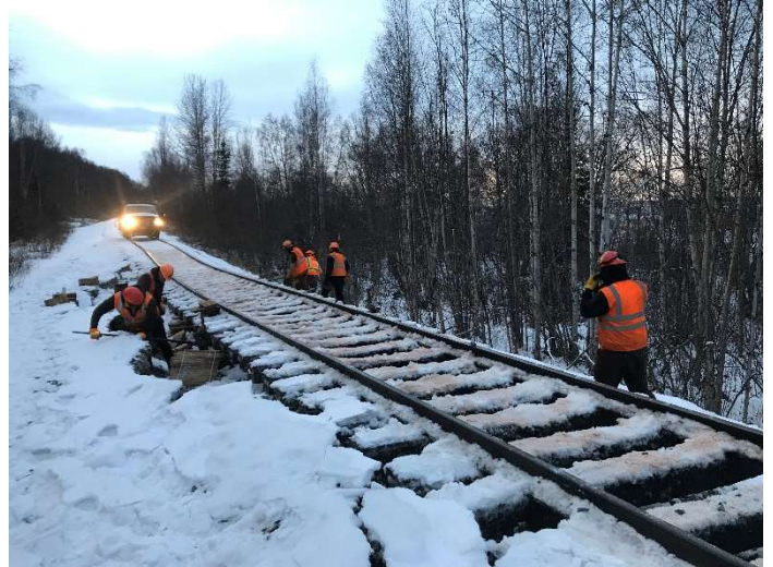
Photo 2: ARRC MOW forces jacking and shimming the affected section of rail at ≈MP 138.5, looking RR South-Southwest.
