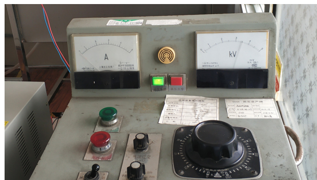
Fig. 7. Regulating transformer test stand.
