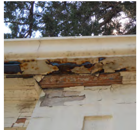
A deteriorated gutter in need of repair.
