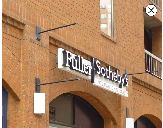
15. Remove remnants of old signage that will not be reused, including brackets and exposed conduit.
