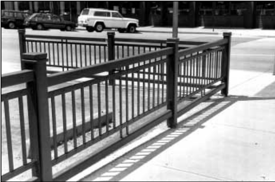
Parking lot railing at 17th Street and Wazee.
