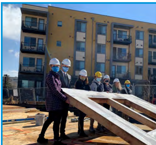
At left: Habitat for Humanity workers raise a wall at the Aria affordable housing development as part of the Carter Building Week. This project will include Aria Apartments with 71 rental units and Aria Cohousing/El Jebel with 8 homeownership units.
