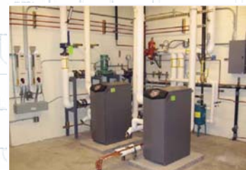
High Efficiency Boilers Save Energy and Building Area.
