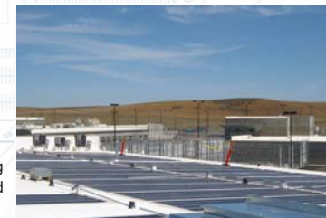
Photovoltaic panels generate power on-site.
