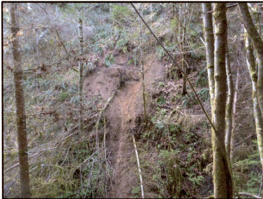
Figure 11. Typical slope along the Creek 2 road location at about Station 18+00 and a recent shallow-rapid landslide from the inner gorge along Creek 2.
