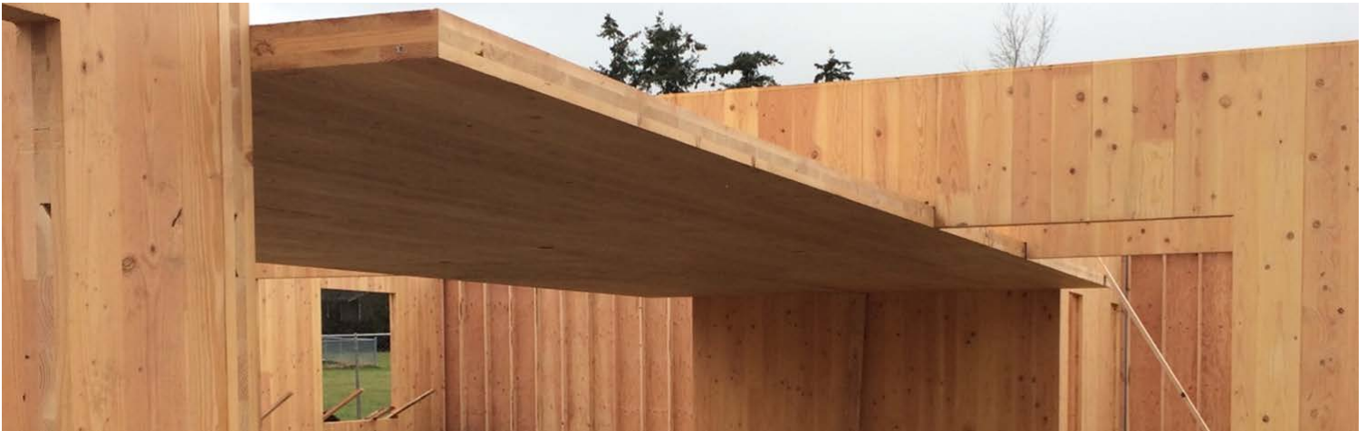
This classroom module, made of CLT panels, was assembled March 7 in Mount Vernon, Wash.
