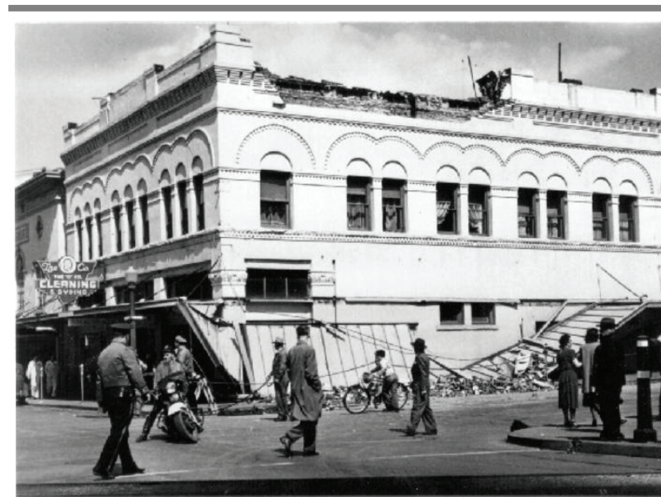
Figure 9. This unreinforced masonry building in downtown Olympia was damaged in the 1949 earthquake. Damage was extensive to this type of building in that event. This building is about one block east of Figure 8.
