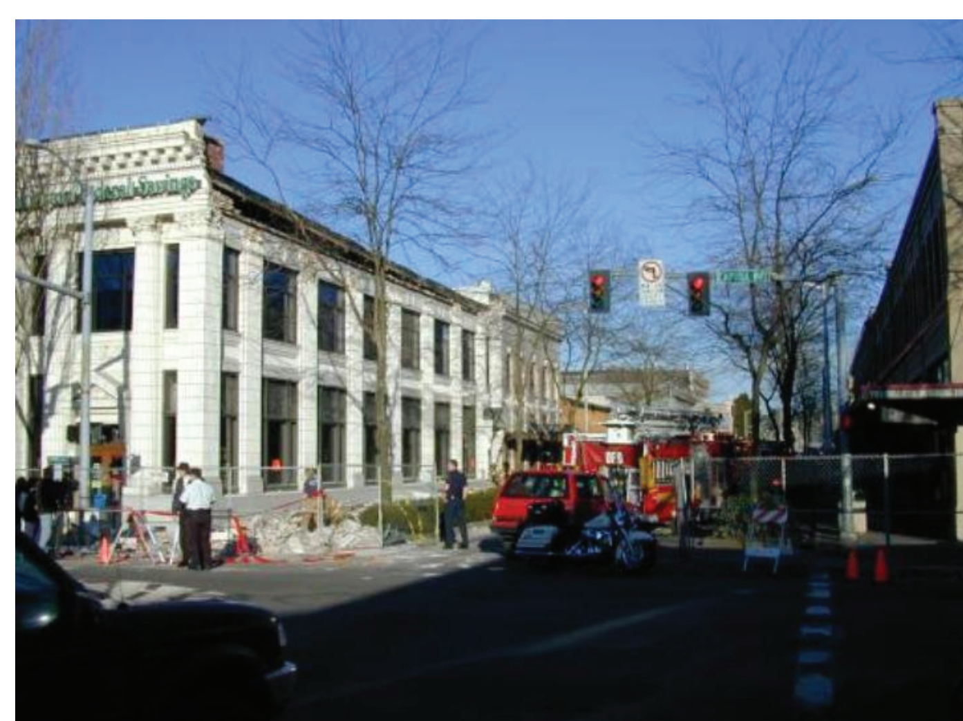
Figure 8. Parapet failure at the Washington Federal Savings Bank in downtown Olympia, which suffered significant damage to older unreinforced masonry buildings.
