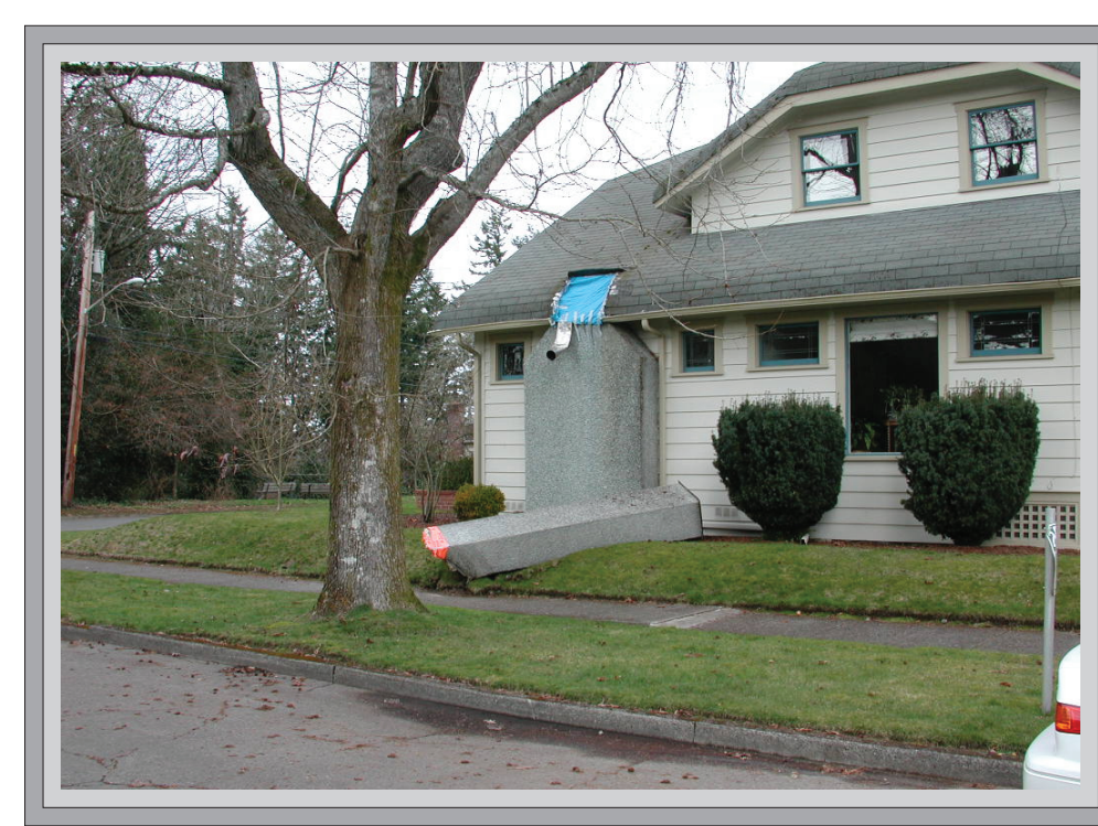
Figure 6. Typical chimney damage in the south Capital neighborhood, where many chimneys were completely destroyed.
