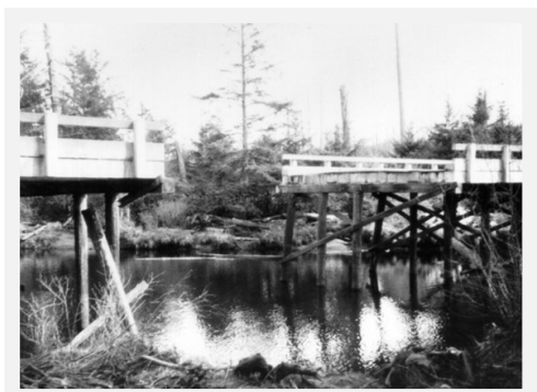
Figure 2: Bridge collapse on State Route 109 over Joe Creek in Grays Harbor County (Credit: U.S. Army Corps of Engineers)
