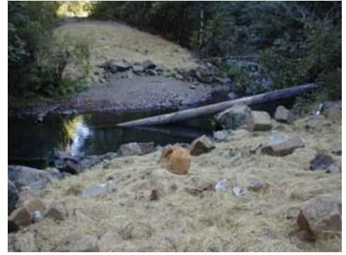
When we abandon outdated forest roads, we restore natural drainage in the former roadbed.
