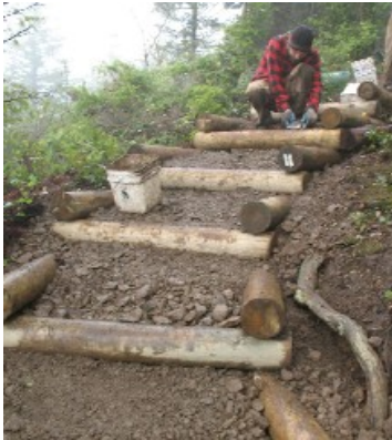
These box steps were built as part of a trail restoration project and will help minimize erosion by providing a water-permeable hiking surface.
