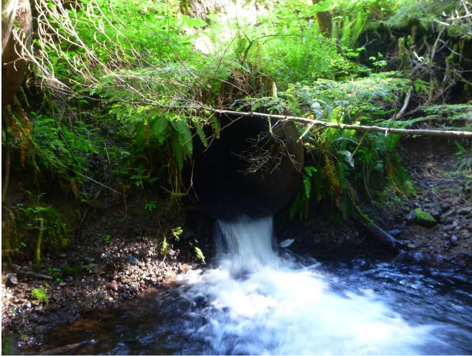
Figure 2. Picture of the Bear Creek culvert scheduled for replacement in 2018.
