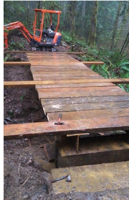
Figure 28: A Bridge in Capitol Forest is Elevated to Reduce Transport of Sediment. Photo courtesy of Philip Wolff.
