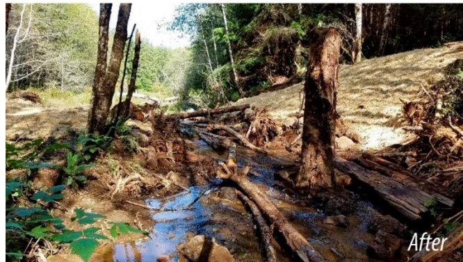
Figure 23: Fish-barrier Removal on Nelson Creek, a Tributary to the Copalis River. This project removed two 48” culverts (pictured) and a 36” culvert, and reconstructed an 18’-wide new main channel (pictured) and a 6’-wide side channel. A total of 4.4 miles of salmon habitat were opened up as a result of this project. Photos courtesy of Candace Montoya.
