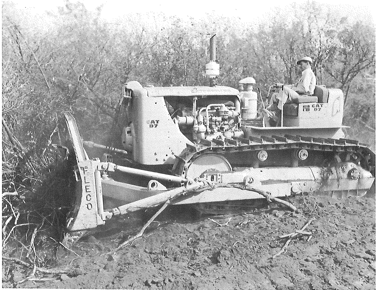
Figure 4. Using a bulldozer with a "root rake" to clear brush from an area to be planted.
