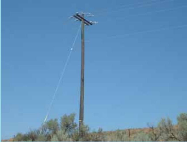
FIGURE 3: 3-phase 12.5-kV line
