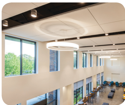
PHOTOS TOP TO BOTTOM: LED high-bays with luminaire-mounted occupancy sensor; touch panel control equipment; daylighting with LED pendant fixtures and track lighting.
