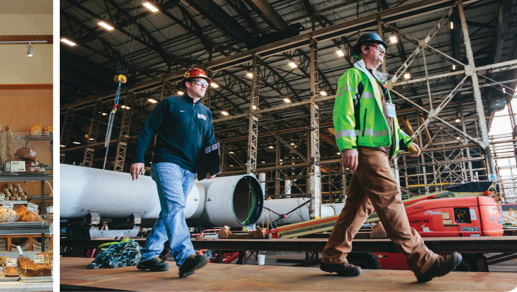
PHOTOS LEFT TO RIGHT: LED downlights and LED accent lights; LED downlights and LED track lights; LED high bay fixtures.
