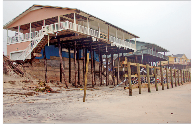
Figure 3-1: Undermined houses constructed on top of the dune in Vilano Beach, FL.
