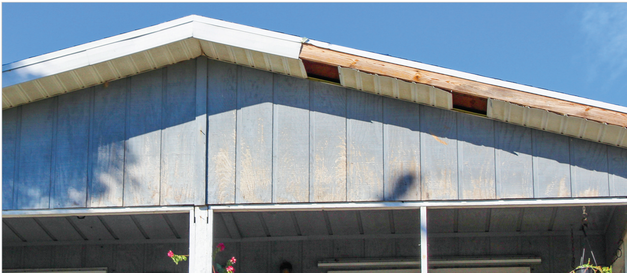
Figure 3-11: House with metal soffit loss below missing fascia cover
