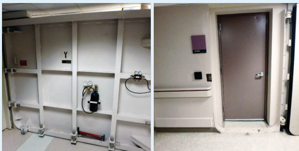
Flood doors in basement that subdivide basement areas within the main building.
