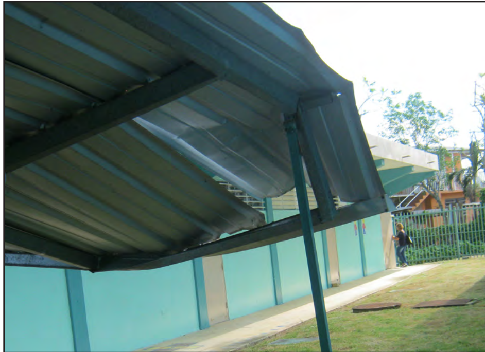
Figure 4-23: Collapsed awning from wind uplift at Jose Robles Otero Elementary School
