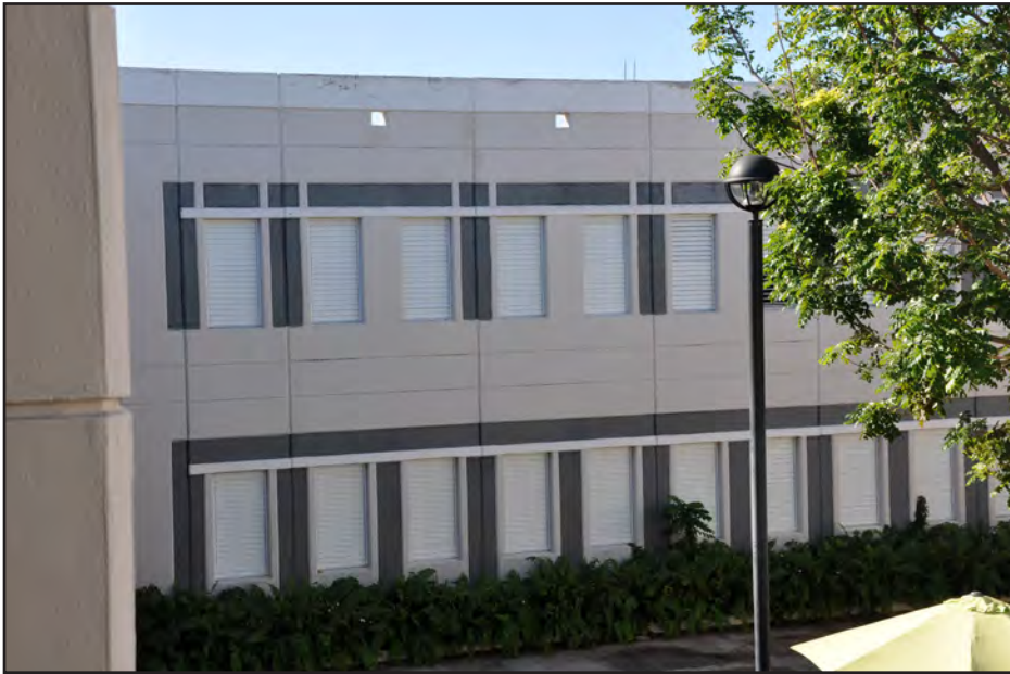
Figure 4-18: Metal panel jalousie windows at Georgina Baquero High School, constructed in 1989. These windows are used across the entire exterior for classrooms and offices. This wing of the school was used as a shelter during Hurricanes Irma and Maria.
