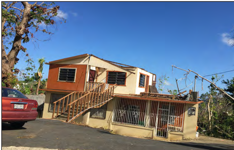
Figure 3-33: Second story wood-framed addition in Canovanas which lost the entire wood-framed roof on the second story addition.
