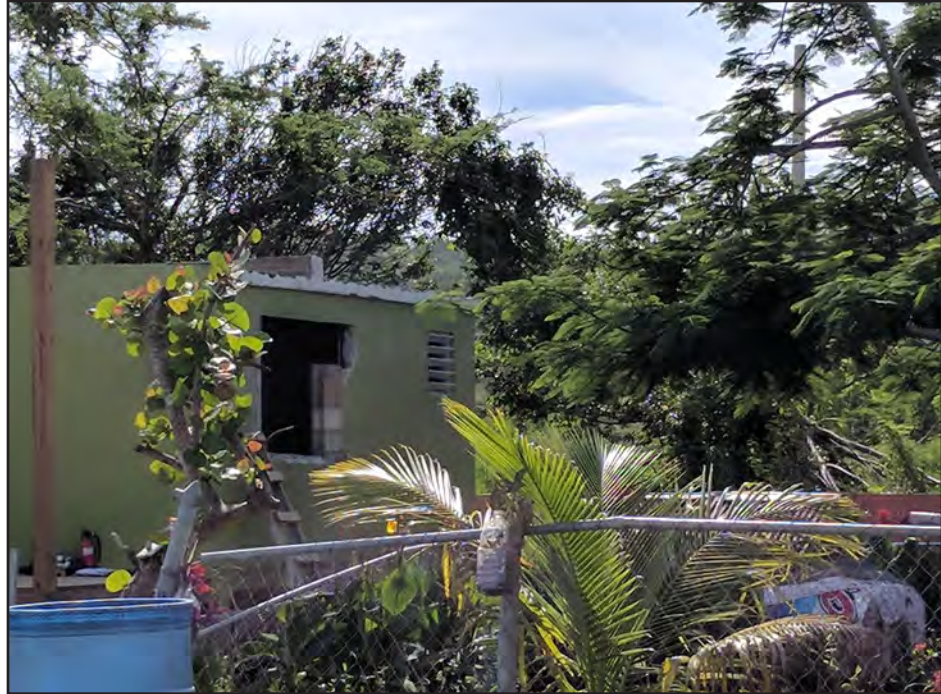
Figure 4-32: This detached residential safe room funded through HMGP in Culebra was modified into a studio/efficiency apartment and no longer complies with FEMA P-361 criteria. Modifications included additional openings which reduced the level of protection provided by the building.
