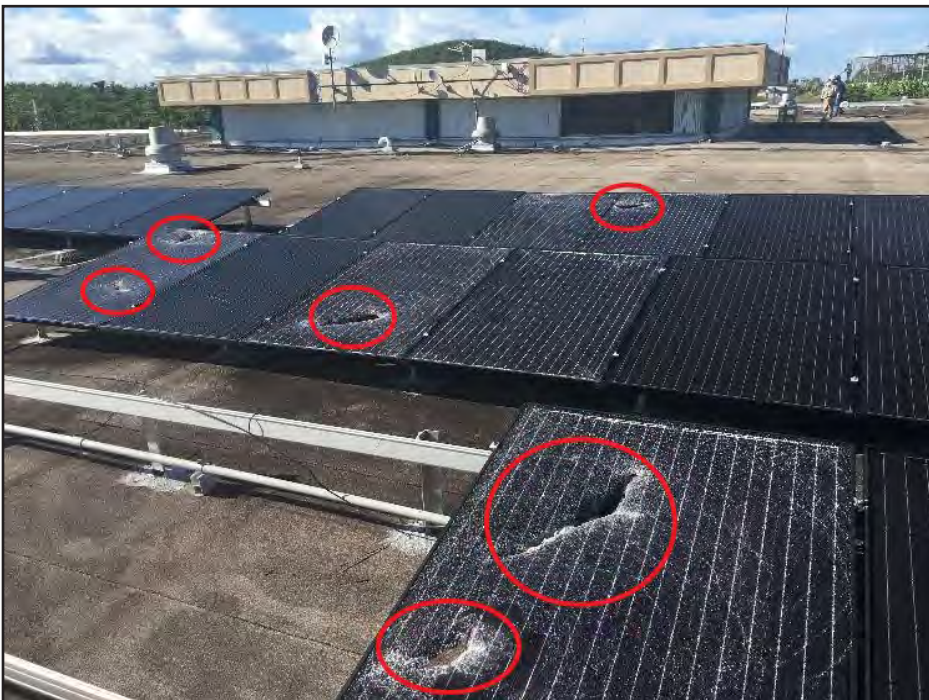
Figure 5-32: Rooftop solar array at east corner of hospital roof showing damage from wind-borne debris impacts (red circles).
