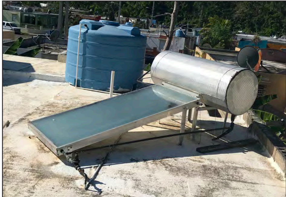
Figure 3-24: Solar water heater and cistern on a residential concrete roof in Rincón.
