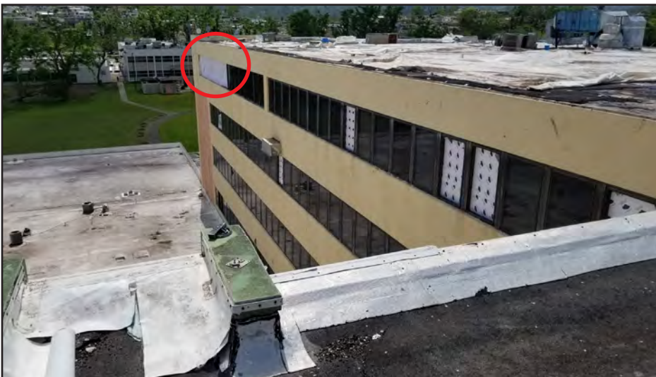
Figure 5-15: View of central section of Dr. Ramon Ruiz Arnau University Hospital showing broken windows as well as entire window and frame missing from wall (red circle).
