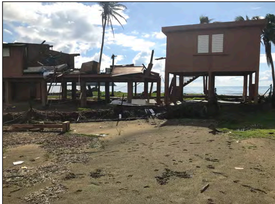
Figure 3-9: Left, an elevated wood-framed house in Punta Santiago was destroyed, right, an elevated concrete house withstood wind and coastal wave forces. Current FIRM: VE Zone.
