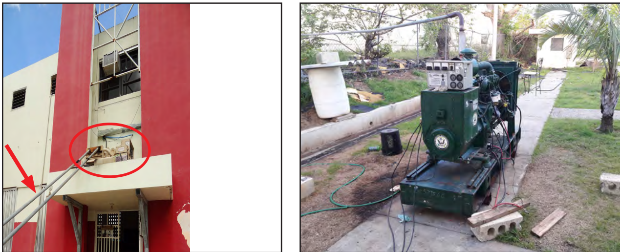
Figure 5-57: Toa Baja Fire Station. Left, generator (red circle) with temporary piping system (red arrow) installed to convey generator smoke away from the building. Right, portable generator supplied after Hurricane Maria.
