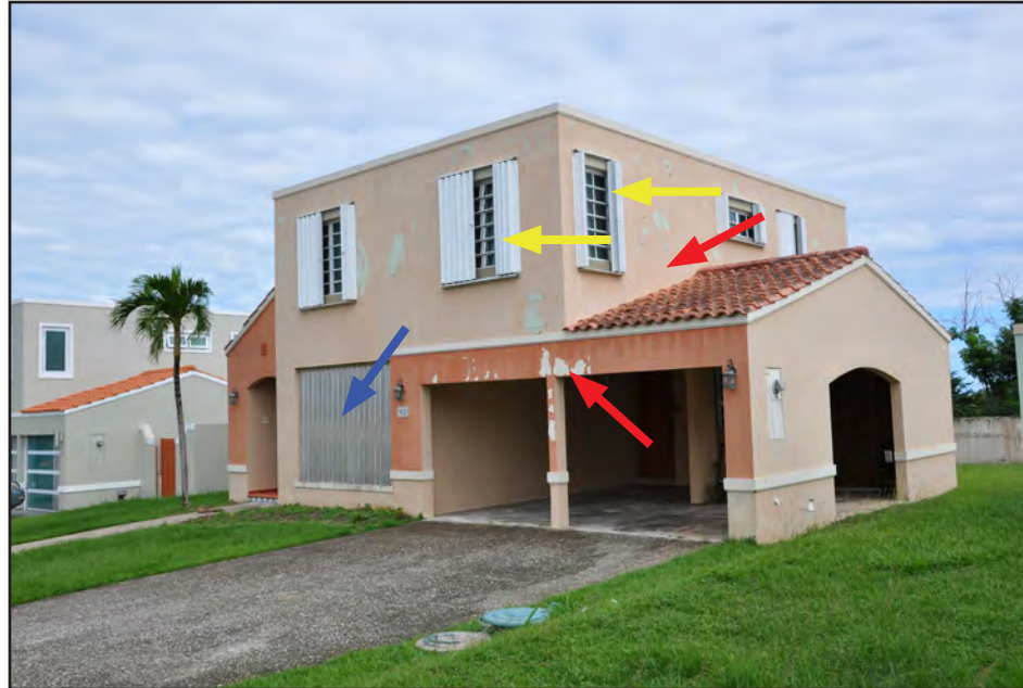
Figure 3-46: Residential building with accordion-style shutters (yellow arrows) on second story over glass jalousie windows and metal panel shutters (blue arrow) on first floor. Glass was protected by shutters, and no windows were broken. Exterior finish was damaged (red arrows).
