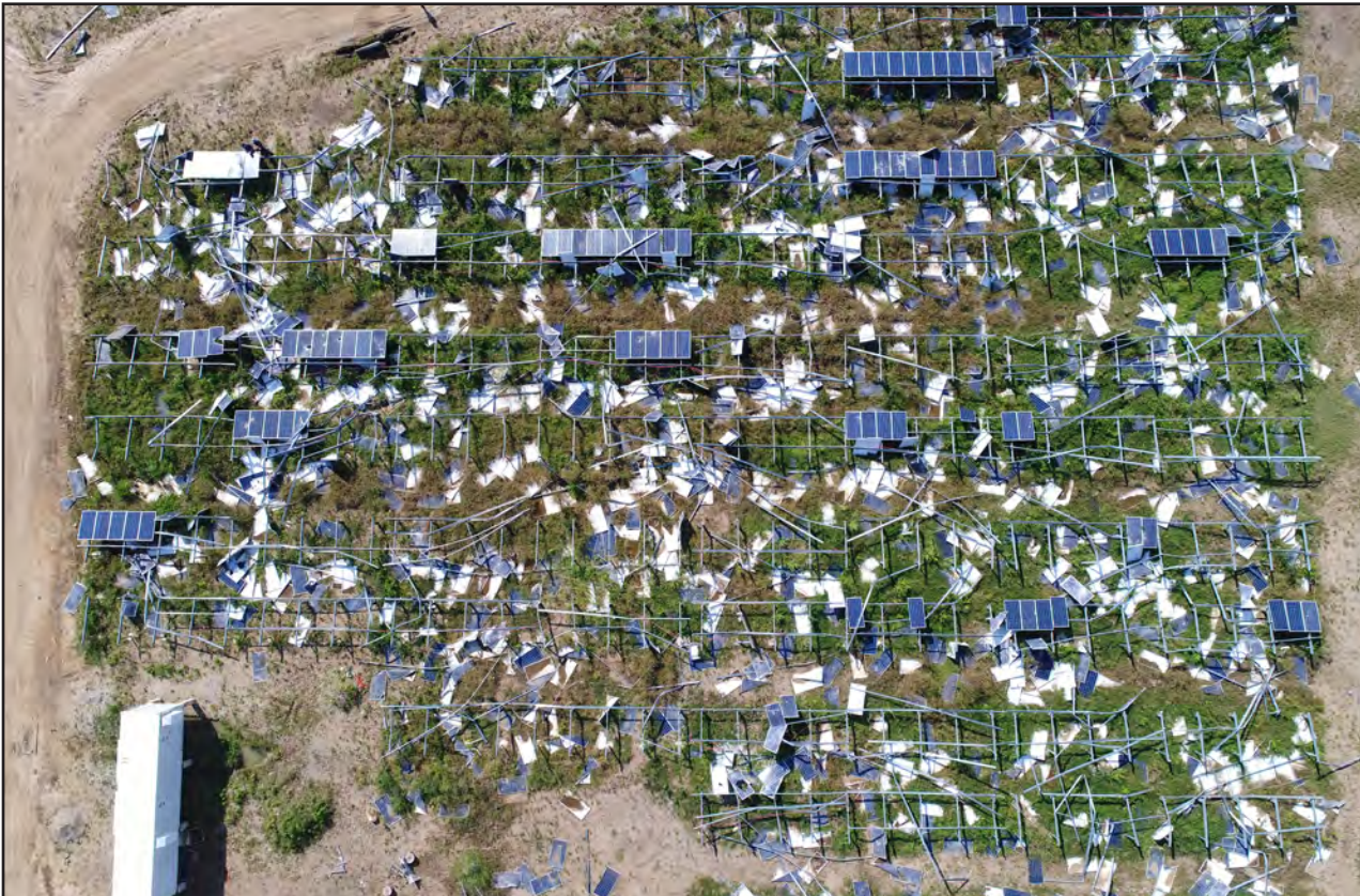
Figure 6-8: Reden solar array in Humacao: Aerial view of the Phase 2 Array with most PV panels removed from their ground-mount supports and many structural members damaged.
