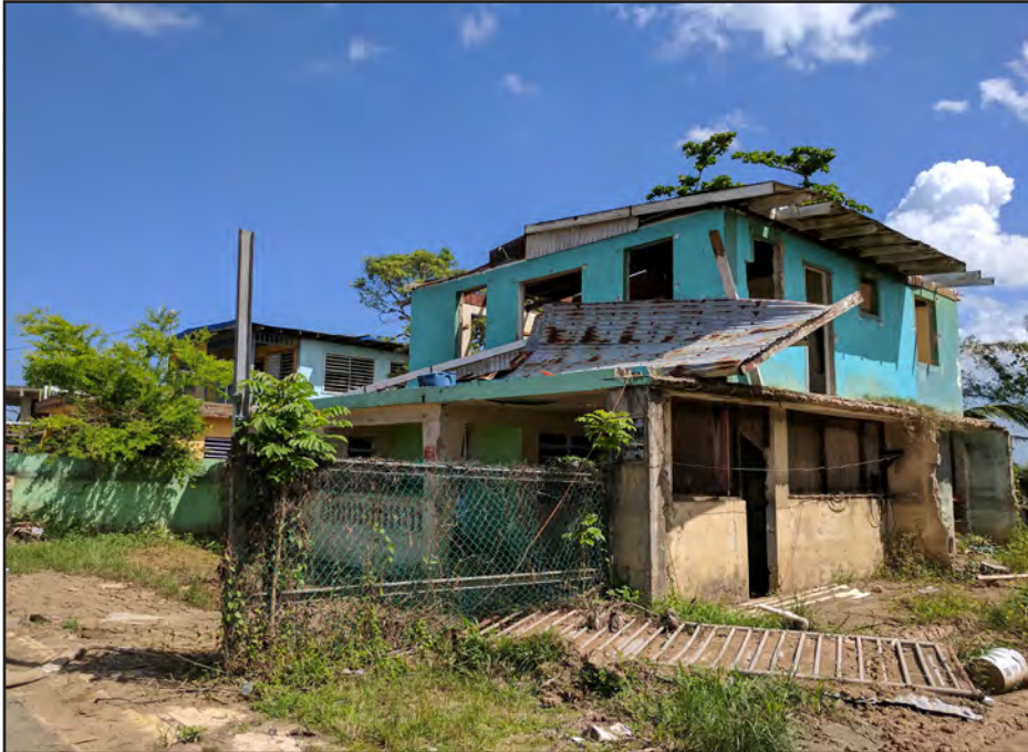
Figure 3-72: Elevated concrete house in Monseratte, Toa Baja subjected to flooding and high winds.
