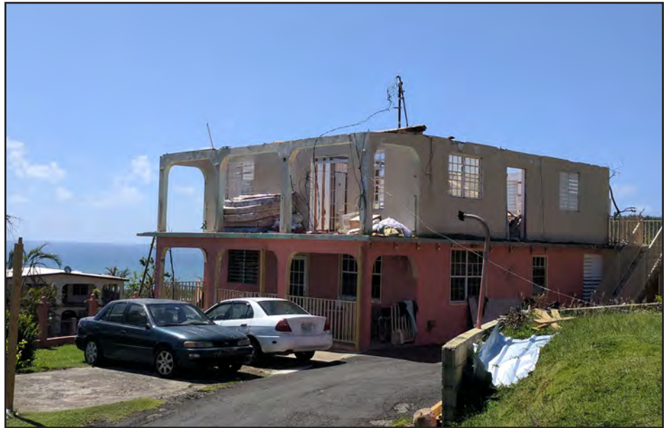
Figure 3-59: Complete failure of informal construction of upper floor structure in Camino Nuevo, Yabucoa.
