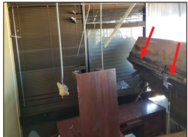
Figure 5-66: Window frames pushed into the PRDOJ building at the top floor due to the failure of frame-to-structure anchors, (red arrows).
