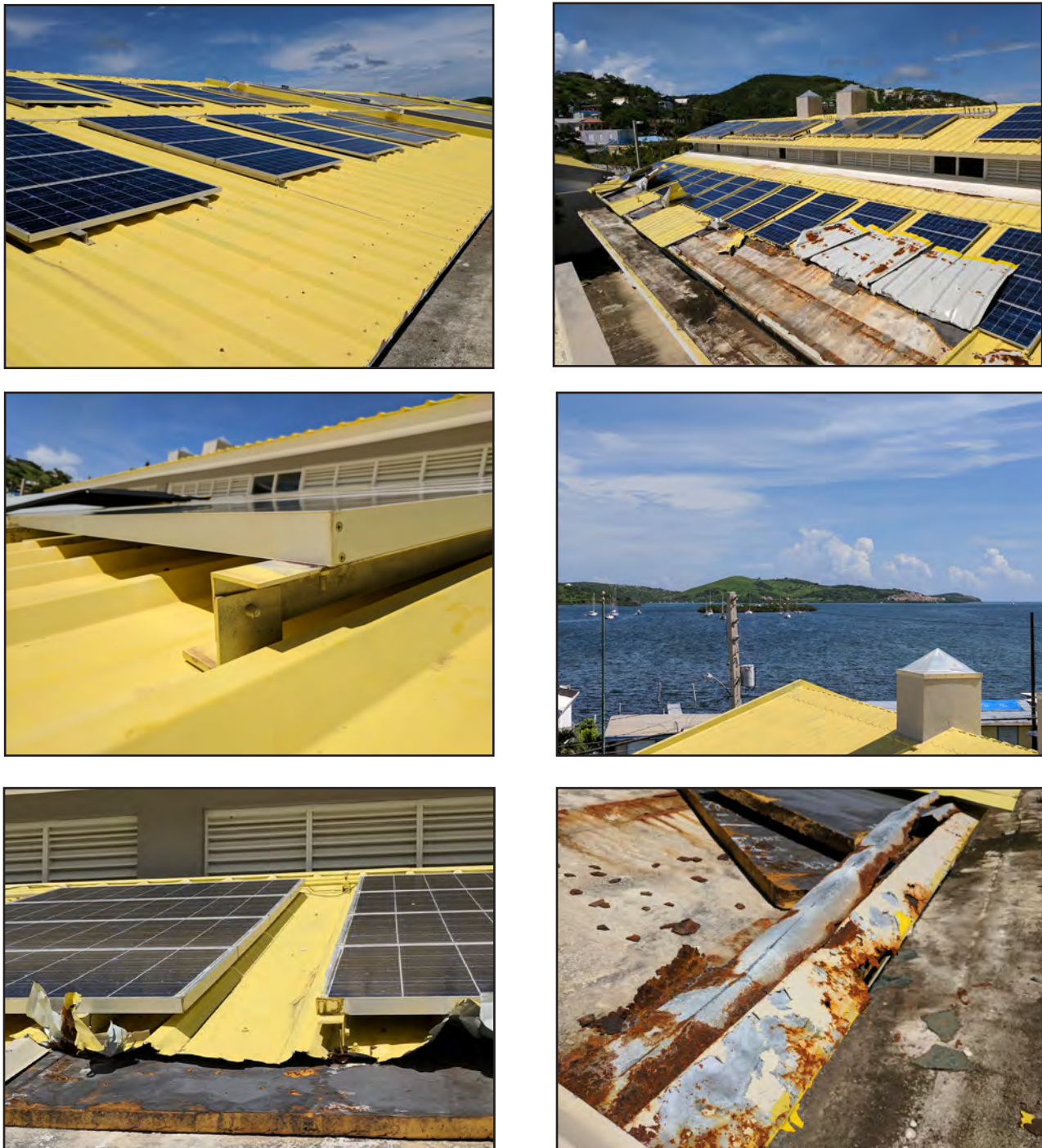
Figure 6-37: Views of the rooftop PV array at Culebra Ecological School, clockwise from top left: undamaged portion of the roof, roof covering failure, close-up of structural aluminum angle anchoring system attaching the PV panels to the concrete roof, open water exposure for the upwind fetch of the intense winds, close-up of failed roof covering section showing exposed rigid insulation foam, view of corrosion on metal roof edge flashing on portion of roof with roof covering failure.
