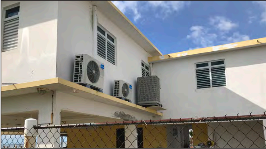
Figure 3-26: Air conditioning equipment elevated on a cantilever at a concrete house in Punta Santiago, Humacao. This means of elevating equipment typically performed well, as here.
