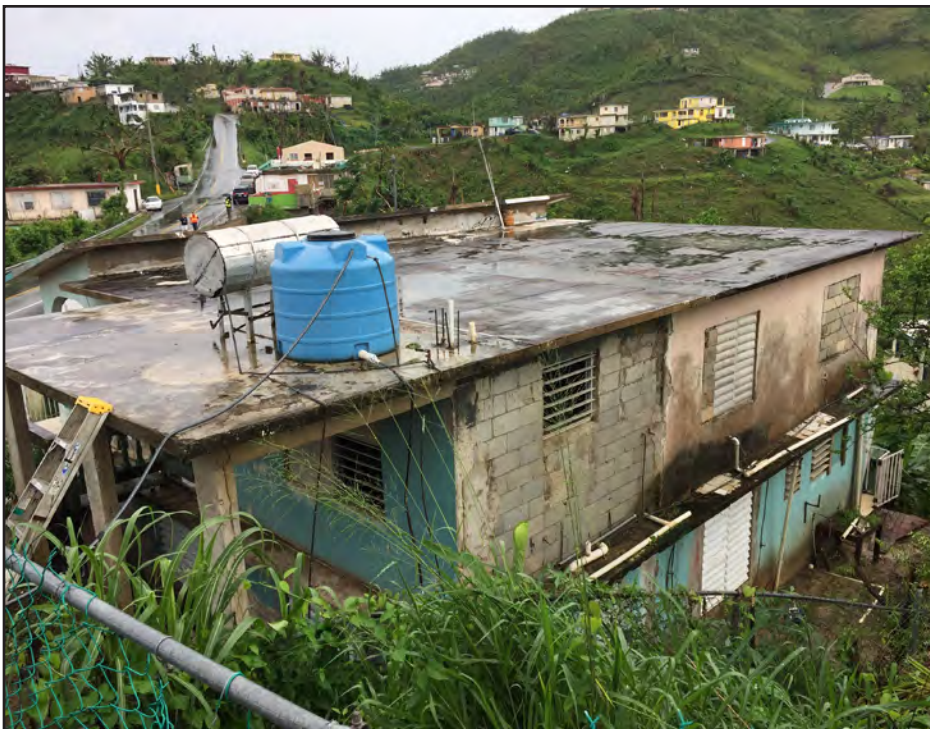
Figure 6-19: Solar water heater system missing solar collector panel on the flat slab concrete roof of a two-story concrete house in El Negro, Yabucoa.
