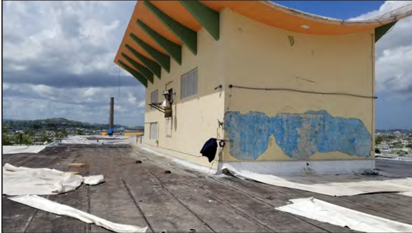
Figure 5-38: Elevator mechanical penthouse enclosing the elevator gear at Dr. Ramon Ruiz Arnau University Hospital. Note ventilation louvers on the sides where rain entered.
