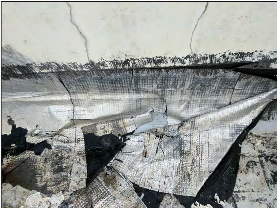
Figure 5-75: Vega Alta Municipal Building had roof leaks. Flashing can be seen displaced at the mechanical area of the roof. Water entered this location as well as others.
