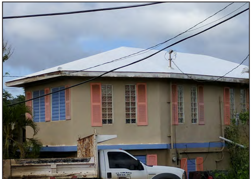
Figure 3-71: This home on Culebra had a plywood roof with a liquid-applied membrane consistent with the Home Protection Roofing Program in the USVI. The roof performed well.
