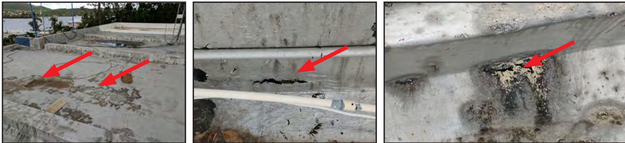
Figure 5-53: Ponding and roof damage (red arrows) at the Culebra Police Station.
