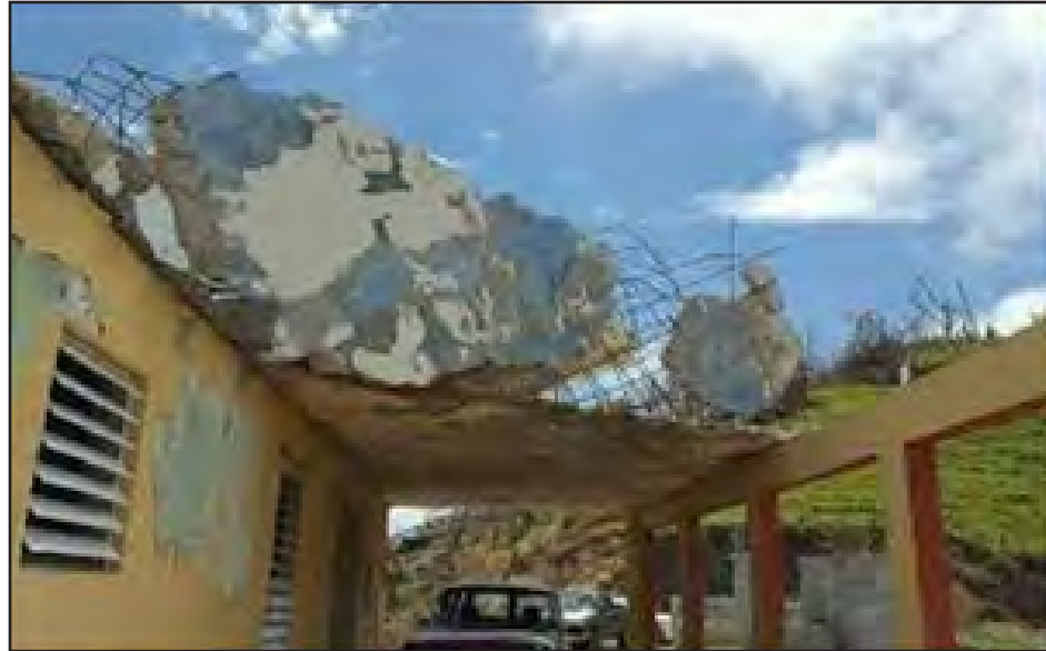
Figure 3-36: Failure of reinforced concrete roof deck over garage. Source: Héctor J. Cruzado, PhD, PE and Gustavo E. Pacheco-Crosetti, PhD, PE.
