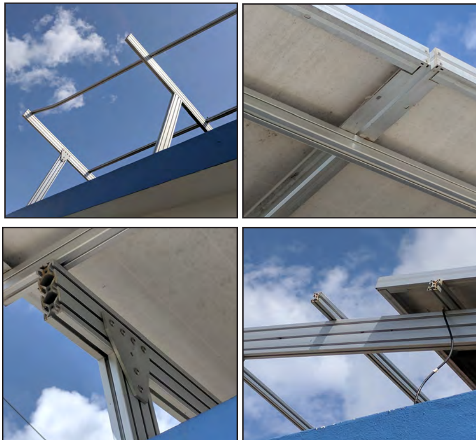
Figure 6-40: Close-up views of the aluminum framing system of the PV power system at Zimmer Biomet facility in Mercedita, Ponce.
