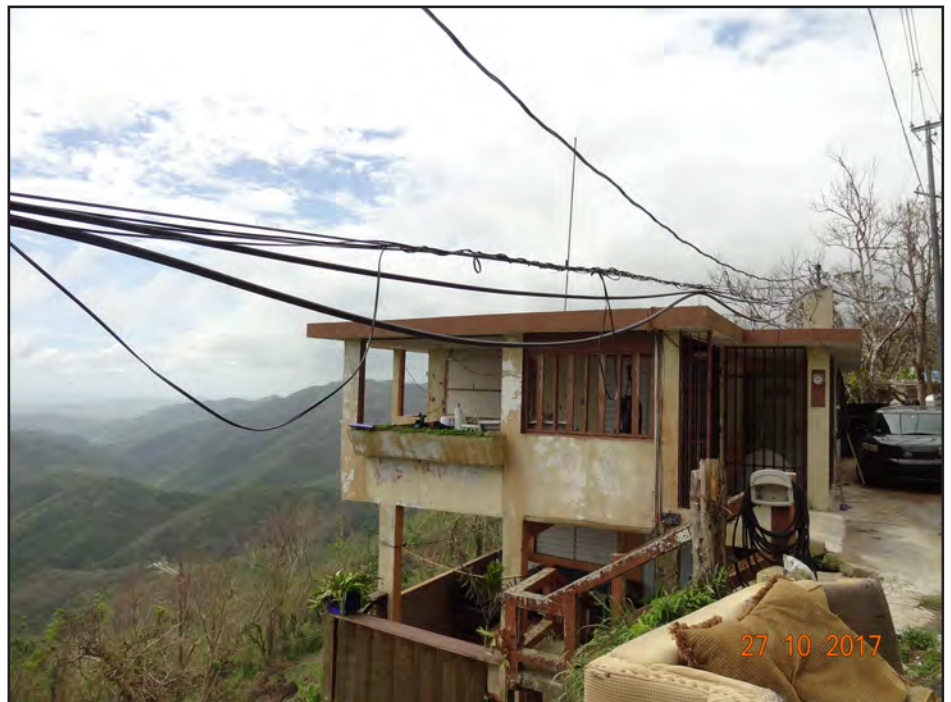
Figure 3-60: Good performance of cast-in-place concrete house set along the steep hillside of Jajome Alto, Cayey.
