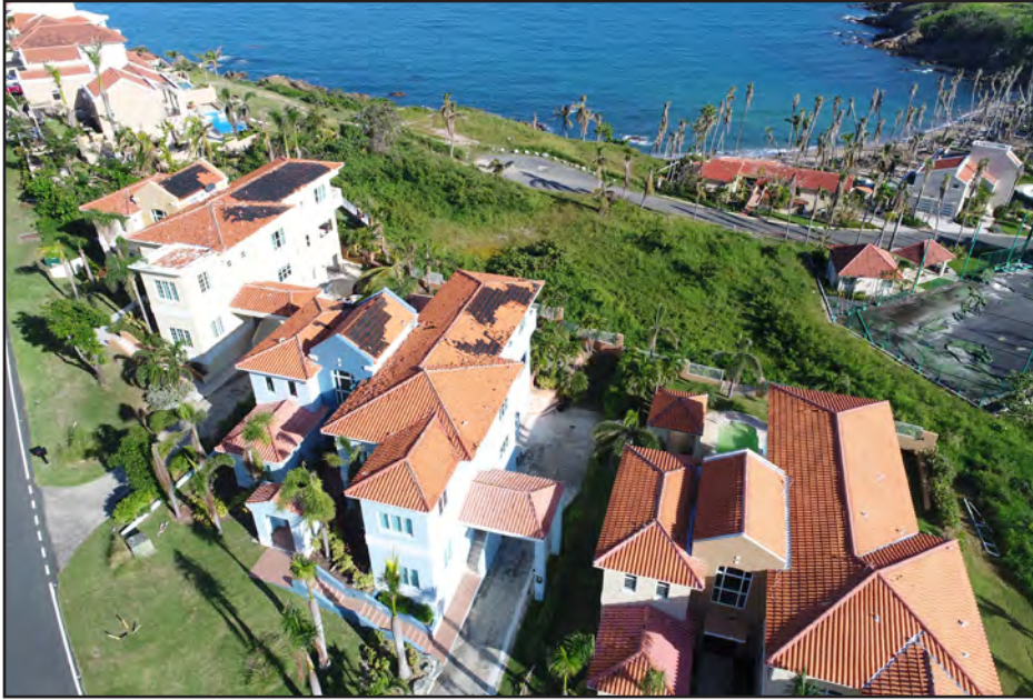
Figure 3-57: Roof damage from wind speed-up effects in Palmas del Mar in Humacao along the eastern coastline.
