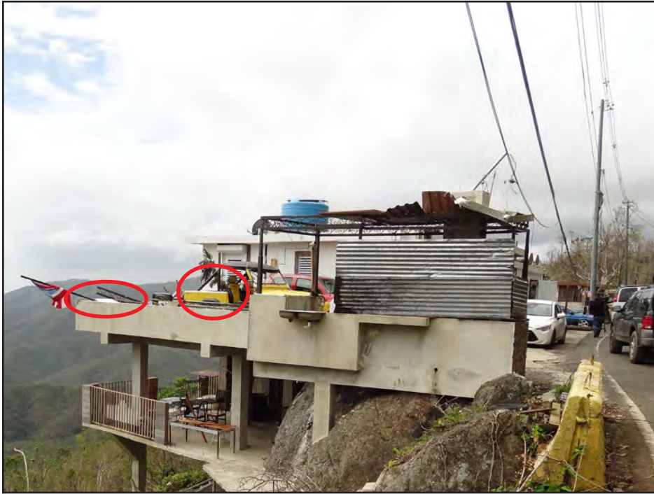
Figure 3-61: Hillside house in Jajome Alto, Cayey. The main building demonstrates good performance under wind speed-up effects, while the informally constructed canopy suffered partial failure (canopy debris, red circles).
