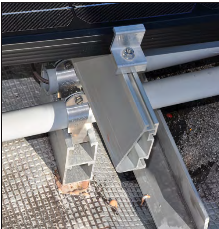
Figure 6-33: Close-up view of the clamping mechanizing connection used to hold PV panels at the edges.
