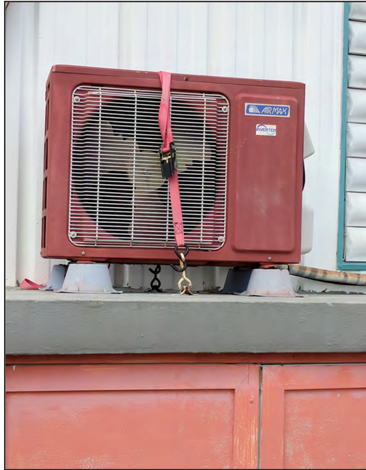
Figure 5-37: This HVAC unit at the Culebra Community Health Center is strapped to a concrete platform; however, it rests on plastic supports that are not mechanically anchored.
