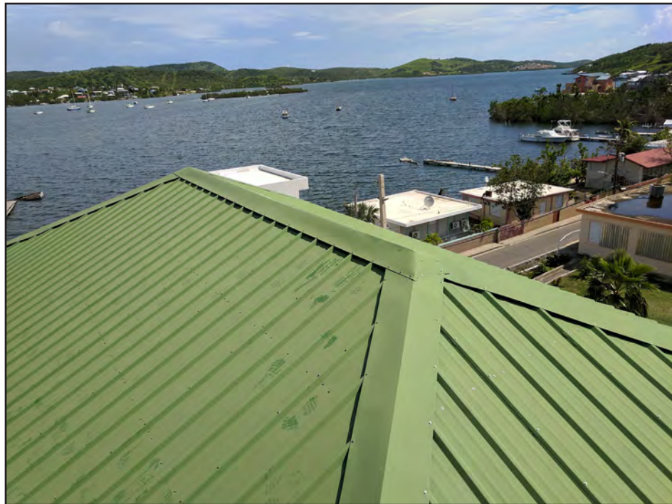
Figure 5-77: Metal roof covering at Culebra Municipal Building performed well. There is no evidence of corrosion from this view.
