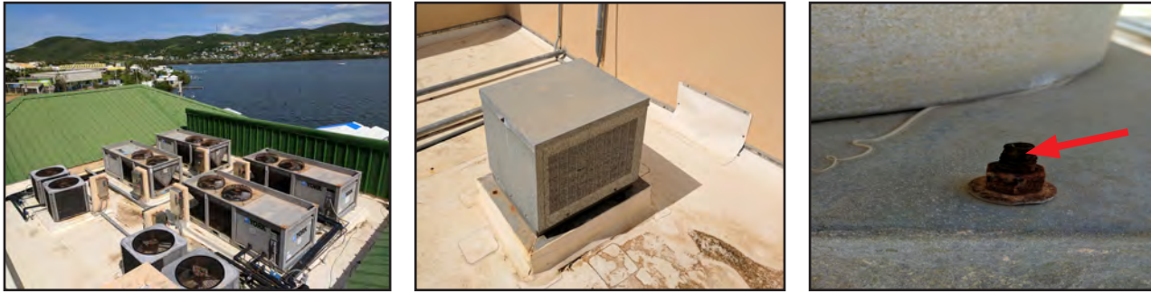
Figure 5-84: Mechanically attached rooftop equipment performed well at Culebra Municipal Building. Some fasteners were corroded (red arrow) but did not fail.
