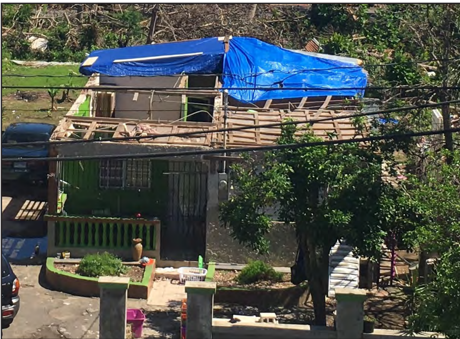
Figure 3-31: Concrete house with major damage to wood-framed roof system.
