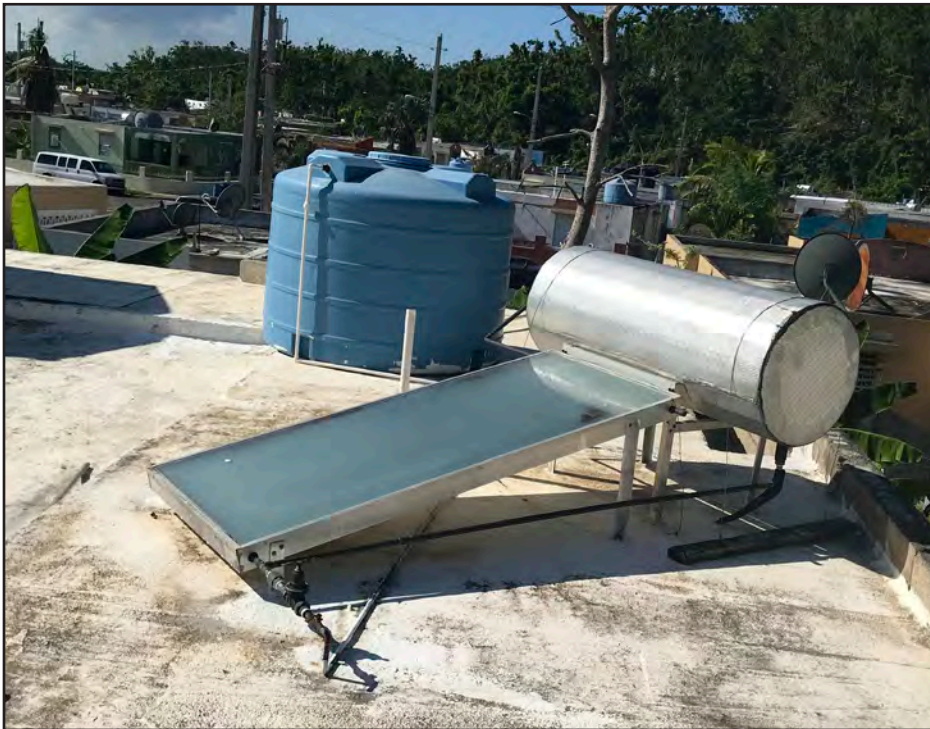
Figure 6-18: Solar water heater unit with flat solar collector panel in Canóvanas.
