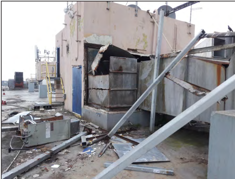
Figure 5-24: Damage to rooftop HVAC equipment at Pavia Hospital Arcibo.
