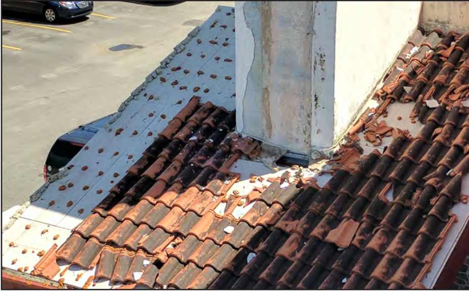
Figure 3-54: Clay roofing tiles inadequately attached to a roof with glue in Palmas del Mar, Humacao.
