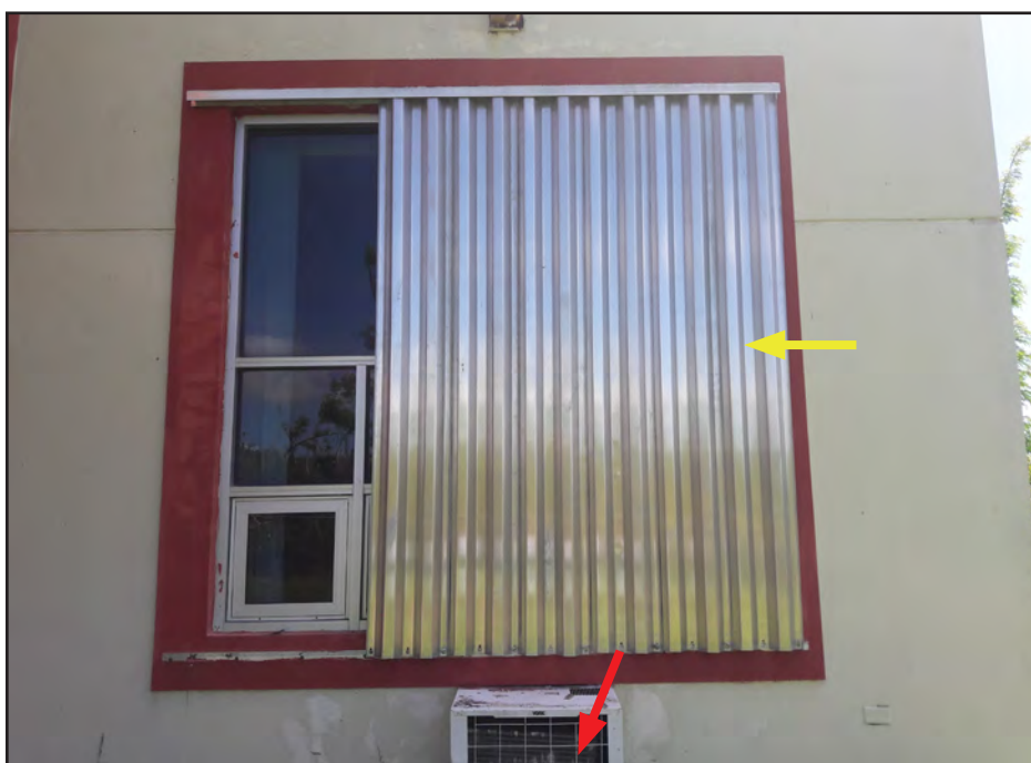
Figure 3-45: Metal hurricane shutter over glazed opening, (yellow arrow). Window unit air conditioner below window was not protected (red arrow) and became a source of water intrusion.
