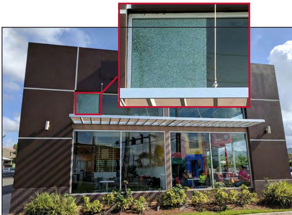
Figure 3-44: Newer low-rise restaurant in Bayamón with impact-resistant glazing panel (red inset) that performed well after being impacted, likely reducing further damage.
