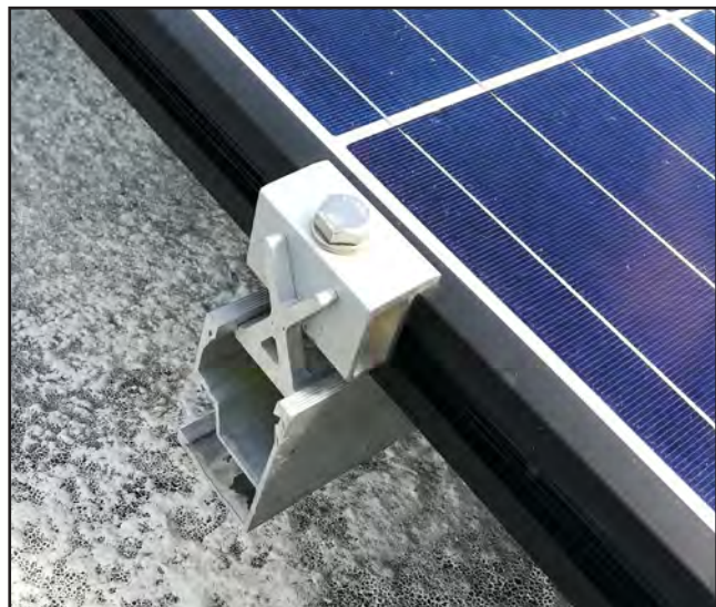
Figure 6-24: Clamp on a PV power system installed on a flat concrete slab roof in Caguas.
