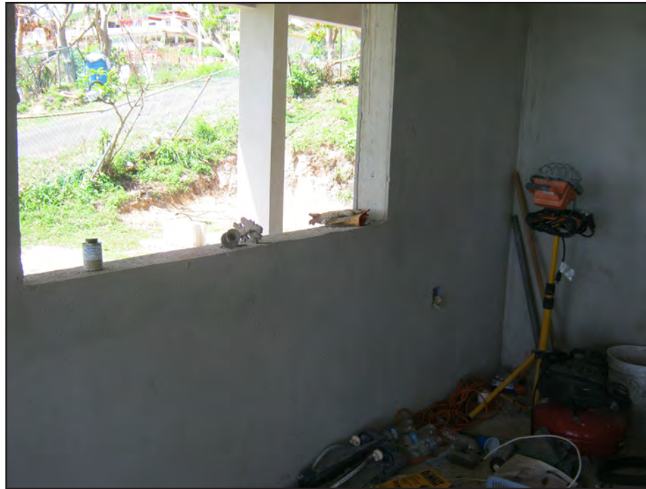
Figure 3-18: Painted concrete, a typical flood-damage-resistant interior finish, in a concrete house under construction in Yabucoa.
