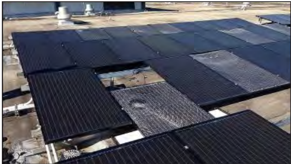
Figure 6-27: PV power system installed at Susana Centeno Family Health Center in Vieques. Close-up view showing PV panels damaged by impact debris.
