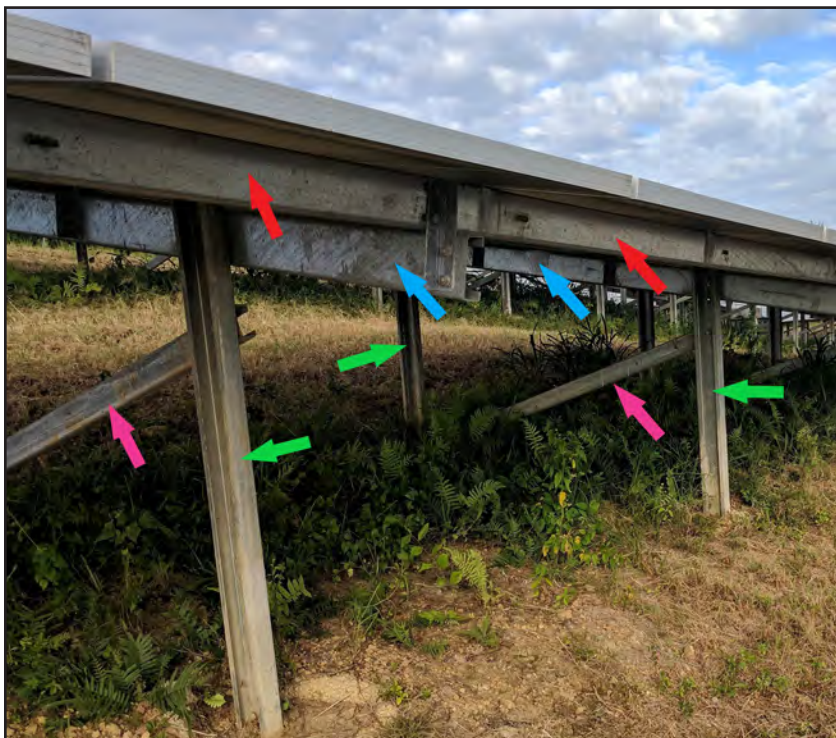
Figure 6-10: Oriana Solar Array 1, showing ground-mounted posts (green arrows), sloped beams (blue arrows), and lateral rails (red arrows), directly supporting the PV panels. This array also has a brace connecting each row of posts (pink arrows).
