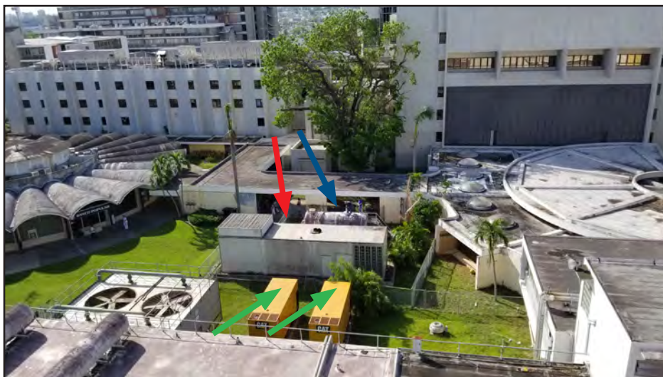
Figure 5-34: View of one of the standby generators (red arrow), two of the backup generators (green arrows), and a fuel tank (blue arrow) at San Juan University Pediatric Hospital.
