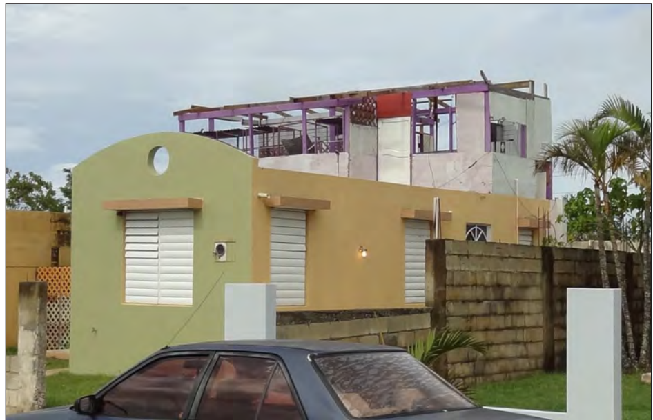
Figure 3-75: NSHP house in Campanilla has an informally constructed addition which lost its entire roof covering.
