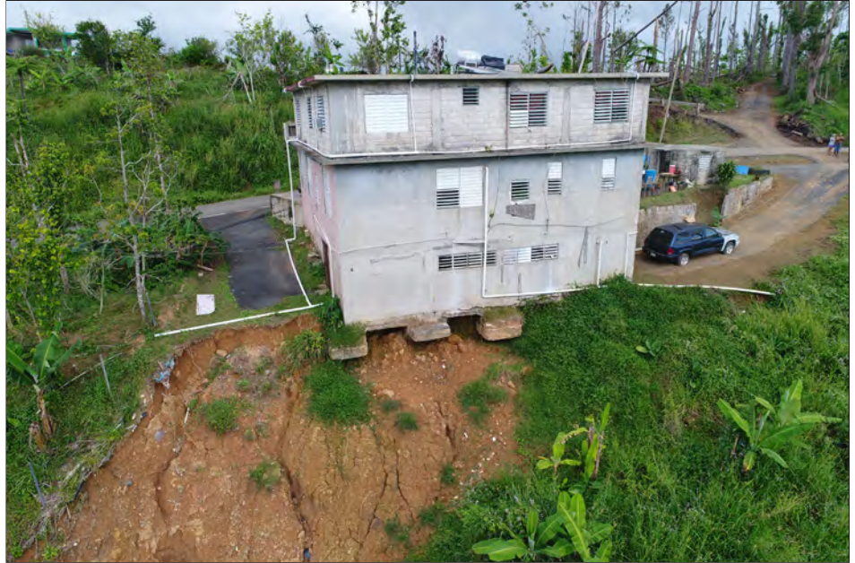
Figure 3-67: Hillside house in Ciales at risk of landslide failure. The house was occupied despite the apparent risk.
