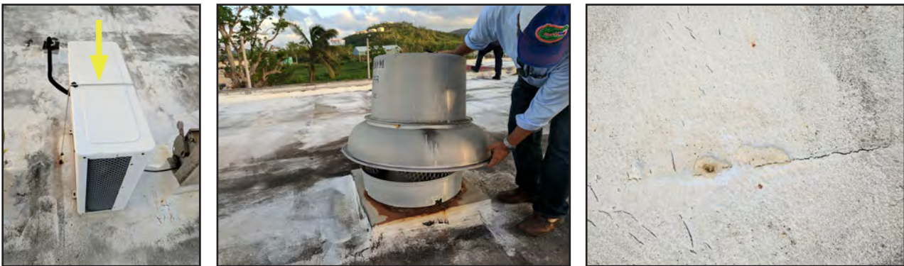
Figure 5-54: Rooftop equipment at the Luquillo Fire Station, including, left, air conditioning unit; center, cooling fan; right, rooftop damage.
