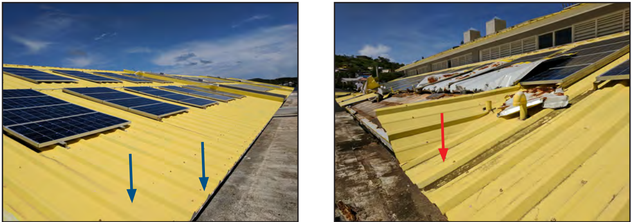
Figure 4-25: Roof covering with two rows of connections near edge of roof covering, left, performed better than roof covering with only one row of connections near edge, right.
