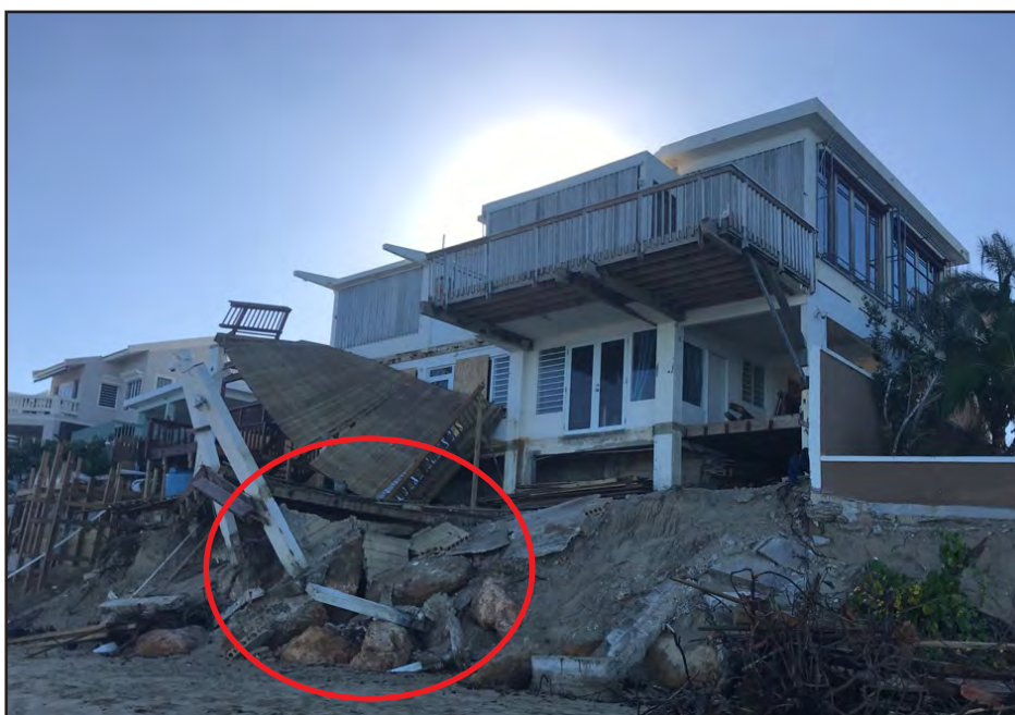
Figure 3-23: Failed CMU wall (red circle) attached to columns at a house in Isabela. The failure contributed to the collapse of a residential deck supported by the columns. Current FIRM: Unshaded Zone X. Advisory Data: Unshaded Zone X, Erosion-impacted area.
