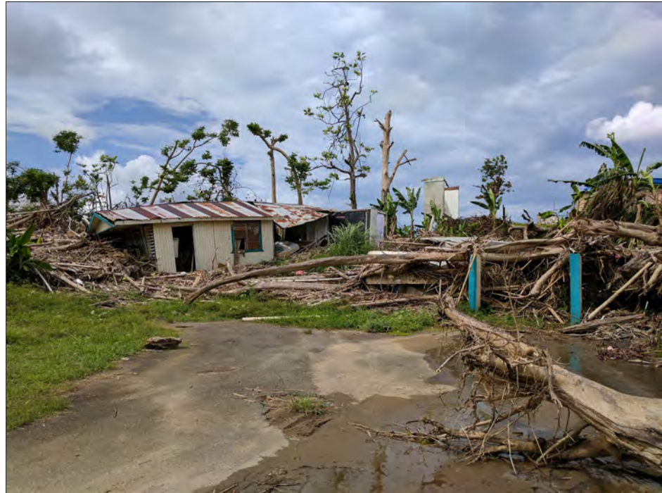
Figure 3-21: Wood framed residence in Toa Baja neighborhood pushed off its foundation by high velocity riverine flooding.
