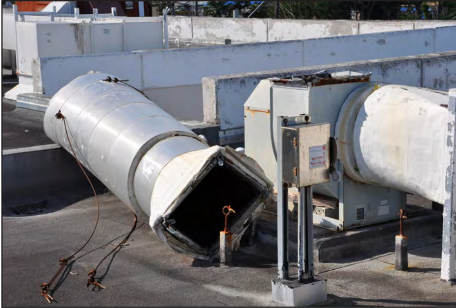
Figure 4-29: Vent stacks secured with guy wires at Loíza Vocational High School were toppled by high winds when the threaded adjustment connectors failed due to corrosion, leading to water intrusion in the building.
