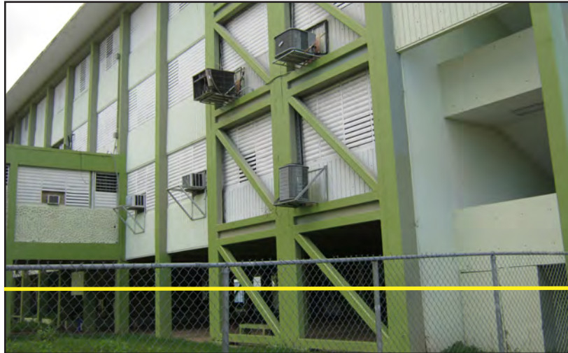
Figure 4-8: Adolfina Irizarry de Puig School building partially elevated with bracing added as seismic retrofitting. Wind damaged these HVAC units. The school received 2.5 - 3 feet of flooding (yellow line).
