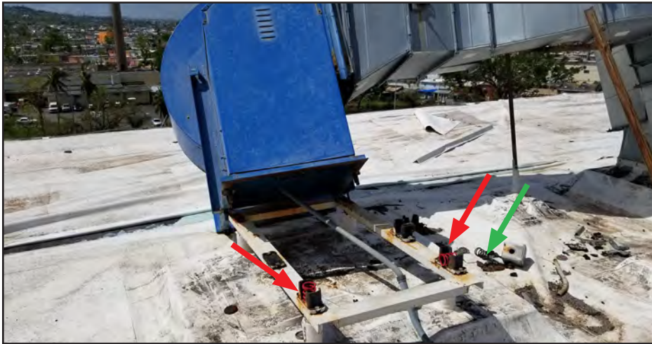
Figure 5-27: Rooftop fan at Dr. Ramon Ruiz Arnau University Hospital displaced from support frame by hurricane winds. Vibration isolation mounts can be seen in the corners (red arrows) and part of another next to the frame (green arrow).
