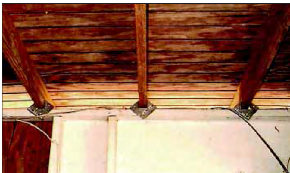
Figure 1-14: Frame connection hardware (hurricane clips) installed in a wood-framed house on Culebra. Source: FEMA (1999a, 52).
