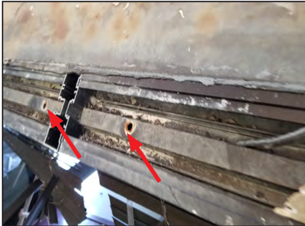
Figure 5-67: View of the undersized anchorage location, (red arrows) in the window frame at the PRDOJ building.
