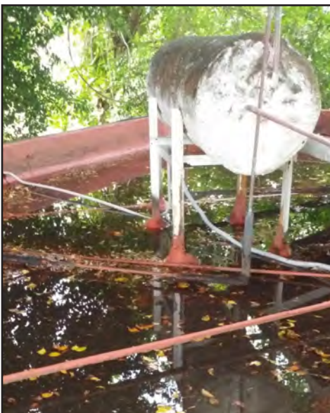
Figure 3-20: Water ponding on flat concrete roof of a residence in San Juan.
