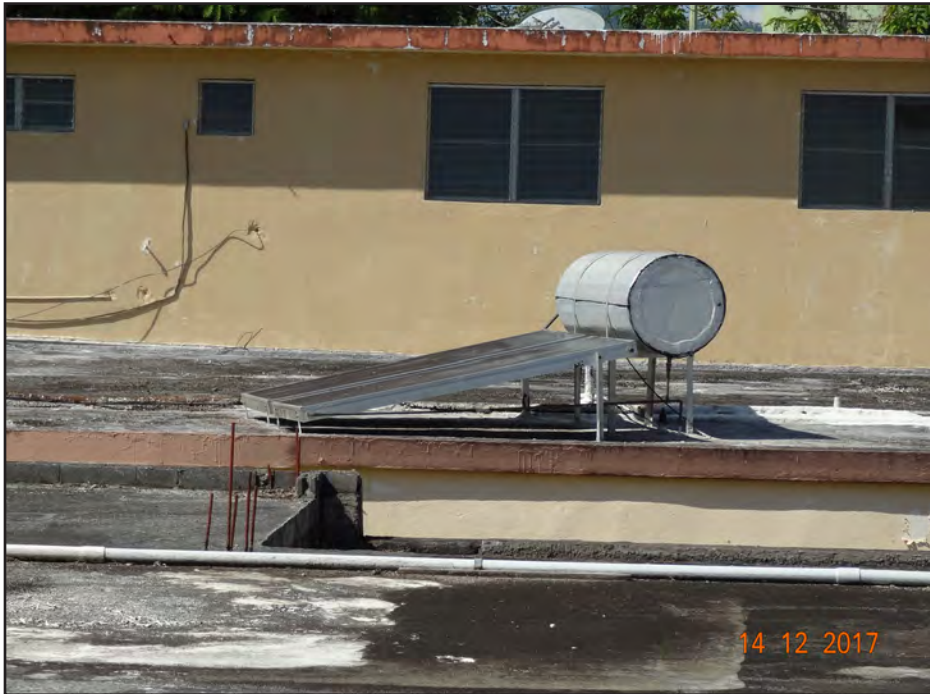
Figure 6-21: Solar water heater system with no evident wind damage on a concrete slab roof of a one-story concrete house in Caguas.
