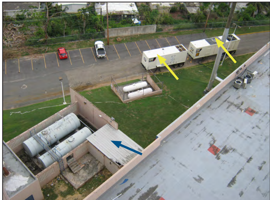
Figure 5-33: Hospital Generator (blue arrow) and two FEMA-Supplied Generators (yellow arrows) at Pavia Hospital Arcibo.
