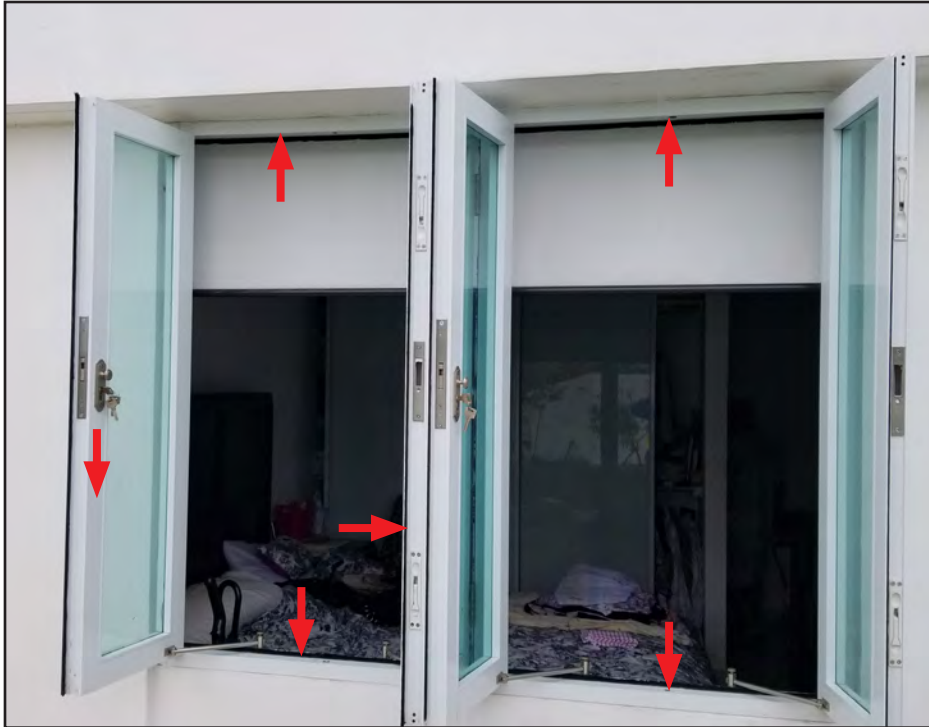
Figure 3-42: Concrete single-family home with casement windows. Windows seal around opening (red arrows) and lock from inside to prevent water intrusion.
