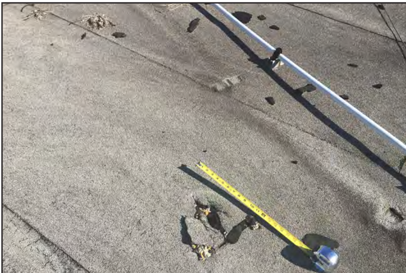
Figure 5-21: Roof covering puncture at Susana Centeno Family Health Center.
