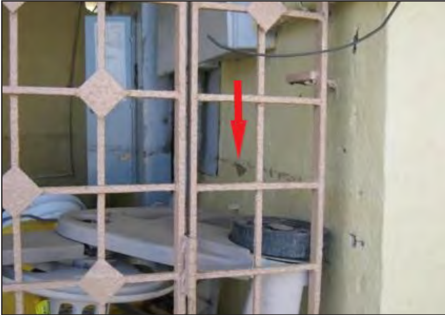
Figure 4-10: High water mark on wall (red arrow) and electrical panel at the Luis M. Santiago School. Flooding of the electrical panel impacted the electrical system across the first floor.
