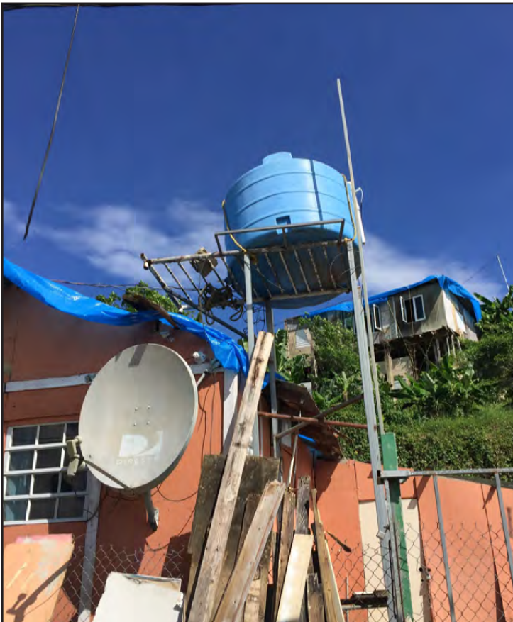
Figure 3-27: This frame supporting a residential cistern did not appear to be professionally designed.
