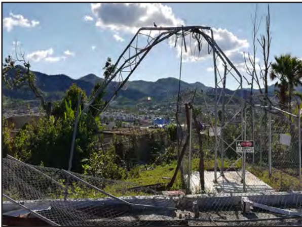
Figure 6-41: Failure of steel communication tower in Cayey.
