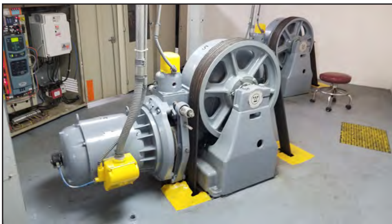
Figure 5-40: Elevator gear and controls located in the elevator penthouse at Dr. Ramon Ruiz Arnau University Hospital.
