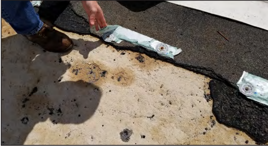
Figure 5-20: The roof membrane at Dr. Ramon Ruiz Arnau University Hospital tore free from its mechanical fasteners.
