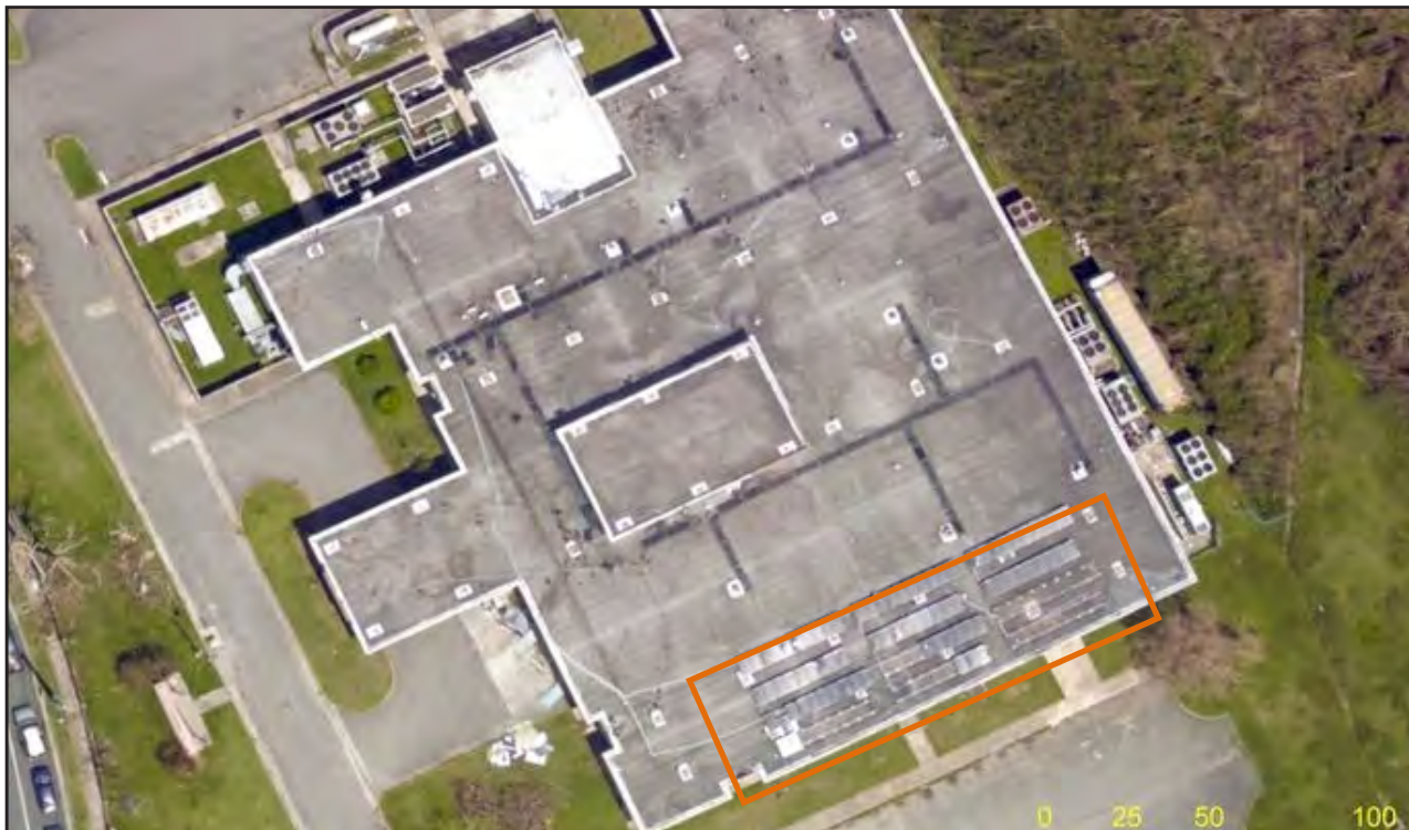
Figure 6-35: PV power system installed on the roof of Susana Centeno Family Health Center, Vieques (Source: aerial image taken September 24, 2017 [NOAA 2017]).
