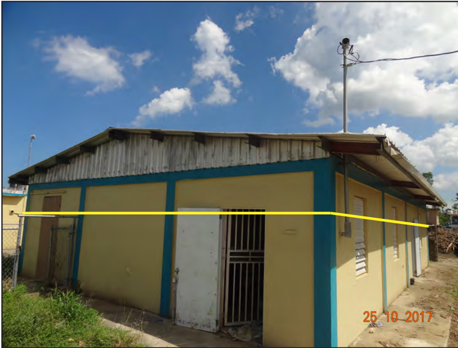
Figure 4-6: Luis M. Santiago School with location of high water mark (yellow line) from Maria.
