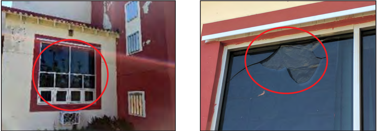
Figure 5-51: The Palmas del Mar community requires decorative tile roofs. The Palmas del Mar Fire Station included decorative tile roof coverings over portion of the building (red circles). The tiles were not mechanically attached, and some failed, contributing to wind-borne debris.
