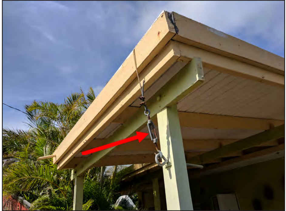
Figure 3-70: A homeowner in Culebra attempted to increase the resistance of the roof to wind uplift forces by means of a steel cable (red arrow) wrapped over roof members and anchored to a column. Such an addition should consider the design loads.
