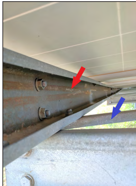
Figure 6-12: Oriana Solar Array 1: The horizontal brace (blue arrow) connecting rows of lateral rails (red arrow) helps distribute wind loads through the structural system and utilize less dependence upon the PV panels to brace the structural system. The horizontal brace also helps resist torsional or twisting action on the ground-mount system.
