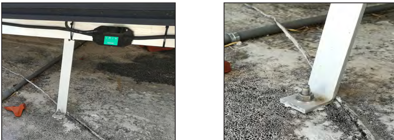
Figure 6-25: Left, PV power system anchored to a flat concrete roof slab in Caguas; right, closeup of bolted connection.
