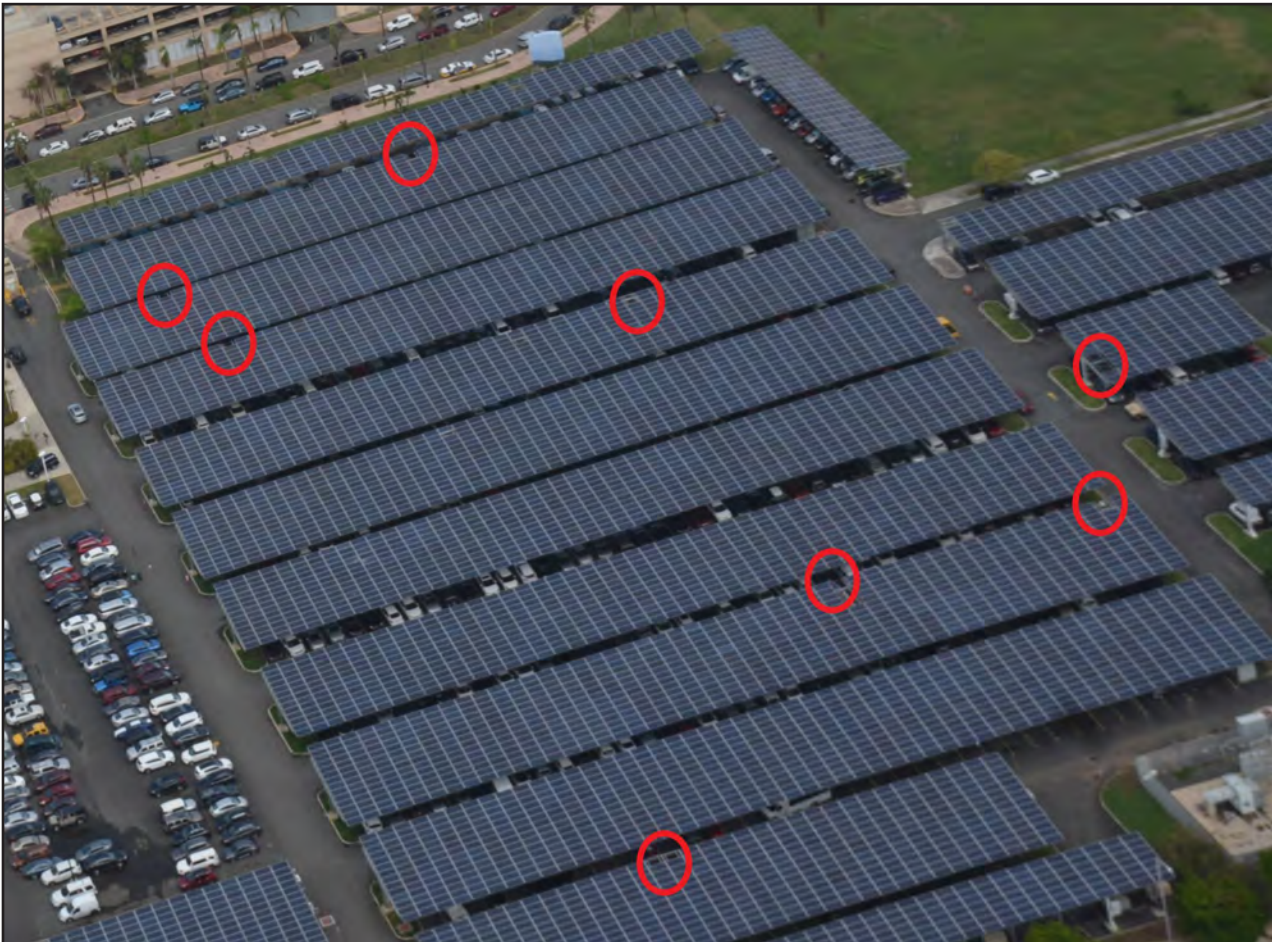
Figure 6-15: Puerto Rico Convention Center Solar Array: Some PV panels were lost (red circles) from these carpports. Based upon aerial imagery, it is estimated that fewer than 5 percent of the panels at this site were damaged or removed (Civil Air Patrol 2017).
