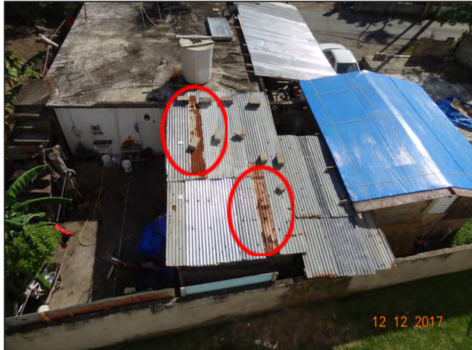
Figure 3-52: House with a corroded metal roof (red circles).
