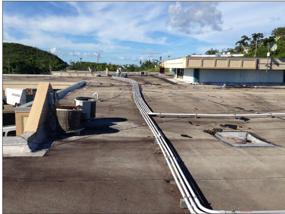
Figure 5-22: View across the roof of Susana Centeno Family Health Center, looking south.
