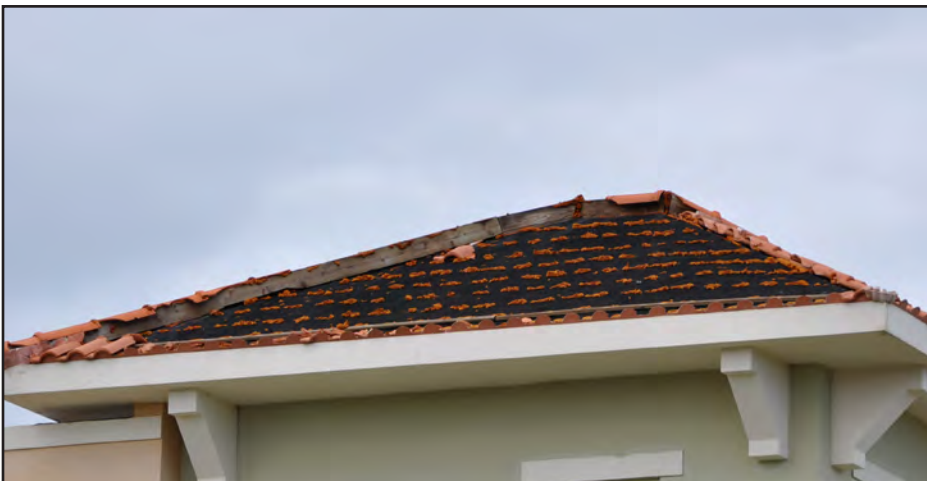
Figure 3-55: Tiles installed on felt over a wooden roof deck. Tiles were removed, but the deck remained in place.
