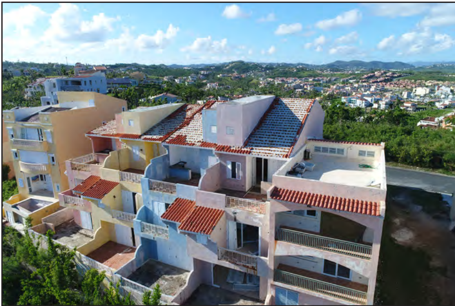
Figure 3-38: Low-rise building on the coast in Palmas del Mar that lost tile roof coverings.
