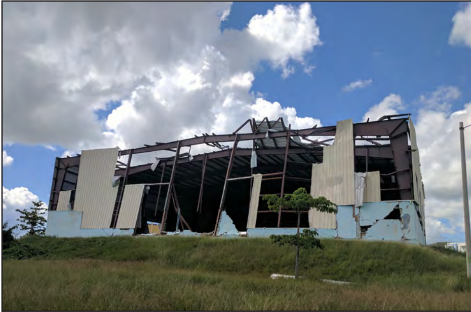
Figure 4-15: The Felix Pedraza Athletic Complex in Ceiba experienced cladding failures and partial failure of its MWFRS.
