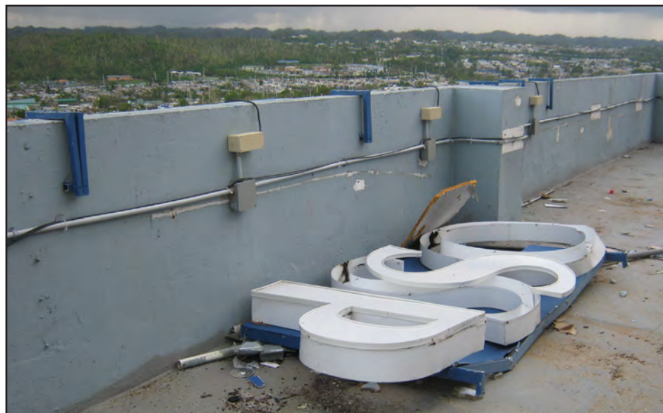
Figure 5-26: Loss of signage at Pavia Hospital Arcibo. The sign frame or armature was inadequately attached to the parapet, and the fasteners failed.
