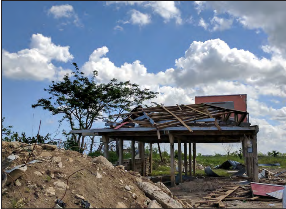
Figure 3-30: Wood-framed house in Toa Baja. With the loss of the roof and wood-framed structural walls, the elevated living space was completely destroyed.
