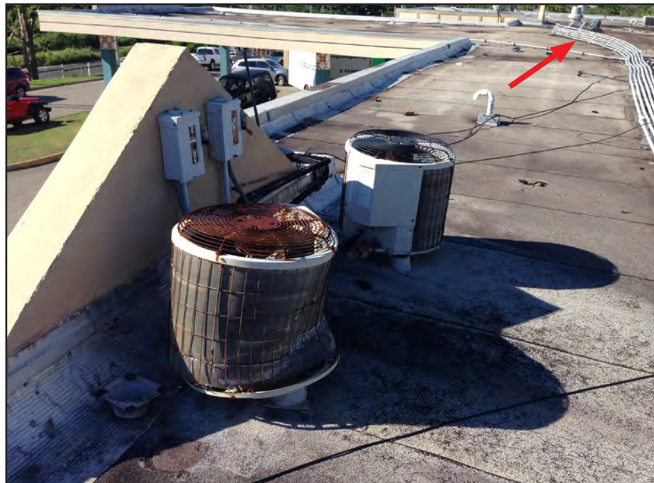
Figure 5-30: Small air handling units displaced and off their stands on top of the roof. Note displaced electrical conduit in background of photo (red arrow).
