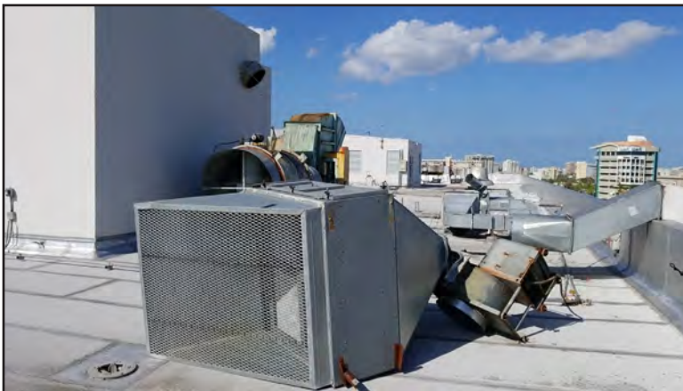
Figure 5-28: Rooftop equipment located on top of one of University Hospital towers that was blown over.
