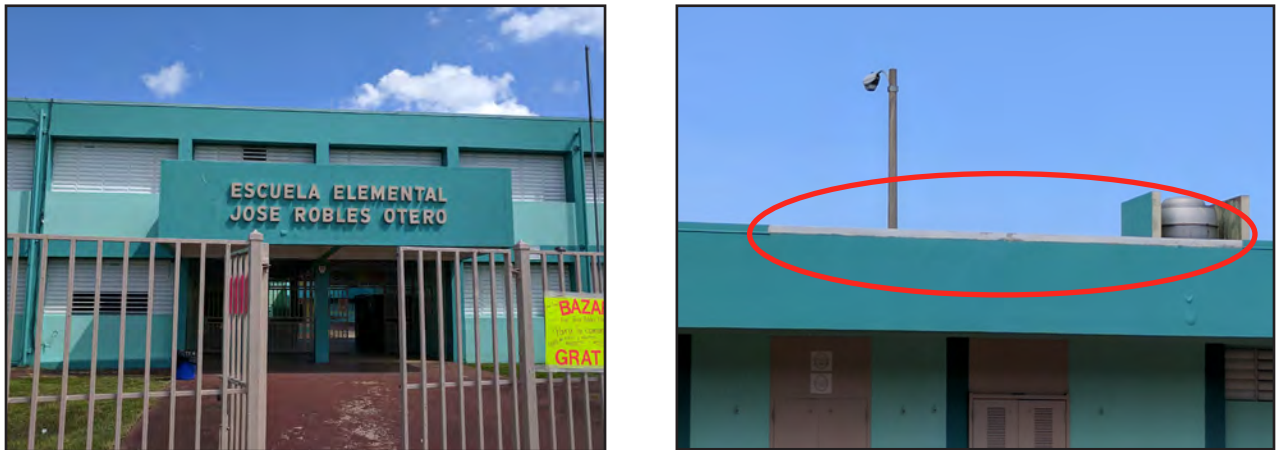
Figure 4-22: Jose Robles Otero Elementary School. Left, façade; right, roof with lost flashing (red circle).
