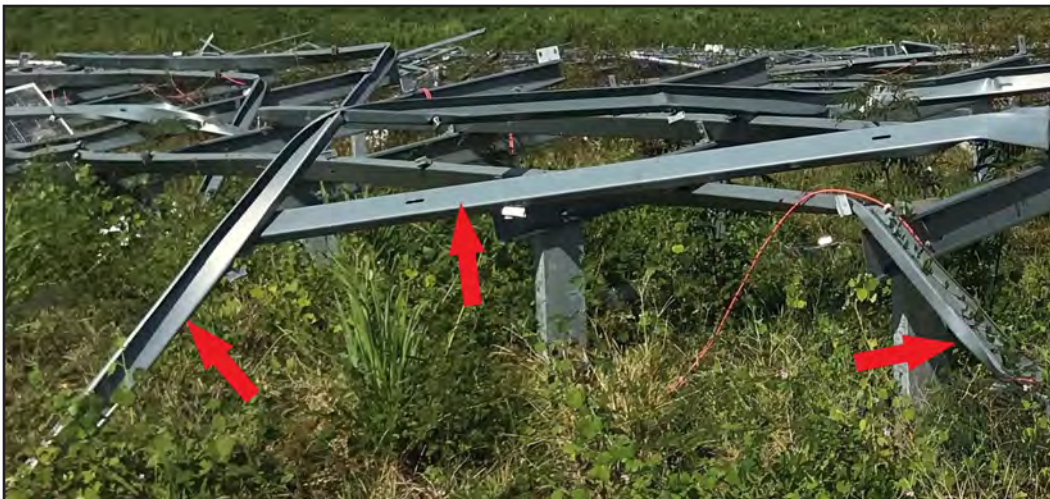
Figure 6-7: Reden solar array in Humacao: Three deformed steel lateral rails (red arrows). In a number of cases the C-shaped lateral rail connections were unable to maintain connection to the steel beams in the high winds.
