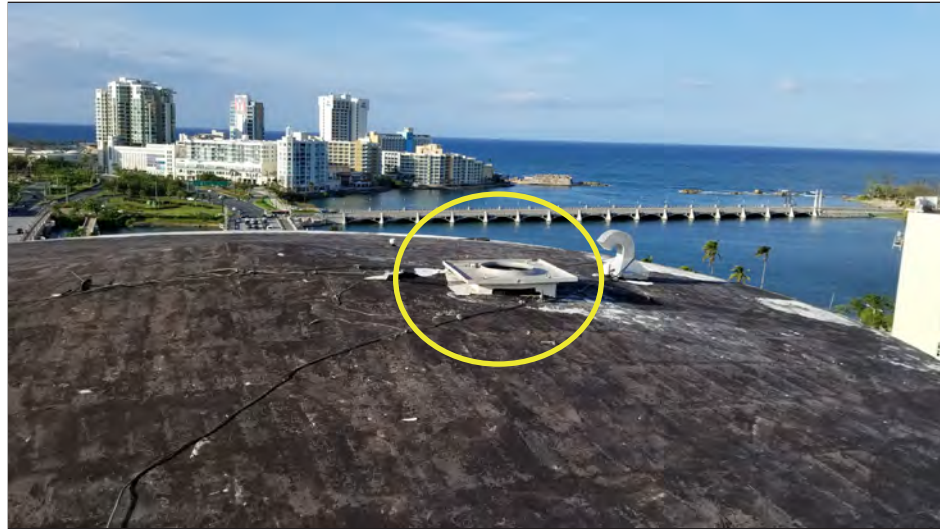
Figure 5-80: A rooftop fan unit is missing from this location atop the PRDOJ building (yellow circle).
