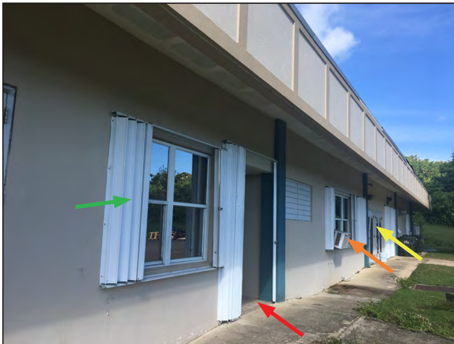
Figure 5-18: Successes and problems related to installation of shutter systems over glazed doors and windows, including a shutter system properly installed (green arrow), a shutter system with a track missing at a glazed door (red arrow), a window air conditioning unit preventing a shutter being deployed (orange arrow), and a pair of glazed doors without glazing protection (yellow arrow).
