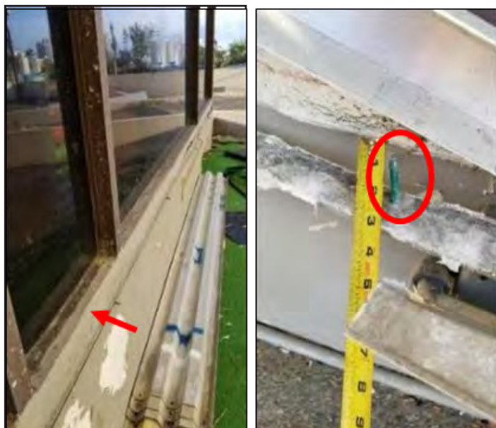
Figure 5-70: Left, shutters protecting lower floor windows pulled off the PRDOJ building, exposing the glass behind; right, the anchors were undersized, of the wrong type, and too few in number.
