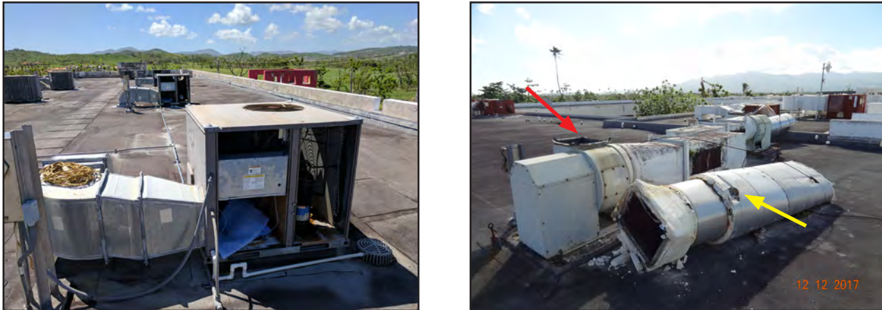
Figure 4-27: Two examples of rooftop equipment failure that allowed water to enter the building. Left, wind removed an HVAC unit access panel at The Palmas Academy. Right, a toppled vent stack (yellow arrow) allowed water intrusion into the building (red arrow) at Loíza Vocational High School.
