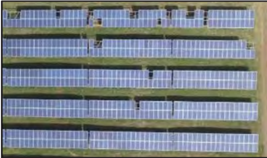
Figure 6-9: Oriana Solar Array 1: Aerial view of one of the more damaged areas within the Oriana Solar Array.
