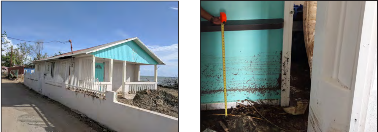
Figure 3-10: Left, house in Playa Cortada subject to damaging storm surge and waves; right, high water mark from storm surge 2.2 feet (0.66 meters) above the floor.
