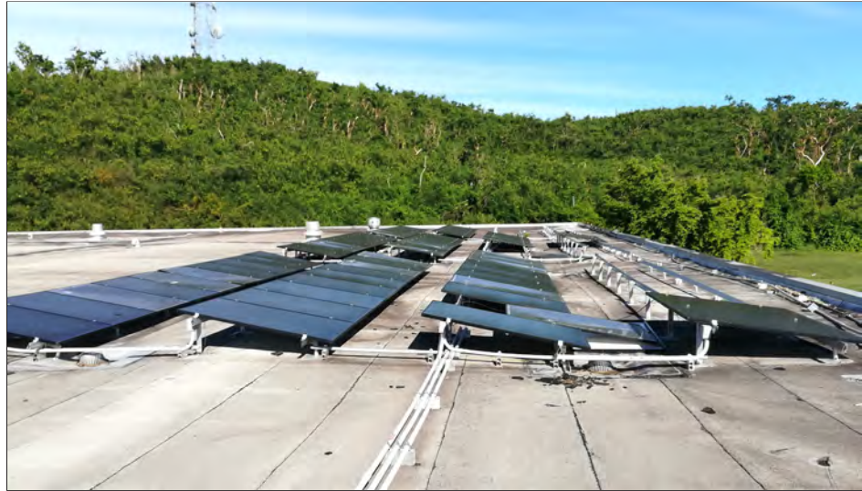
Figure 6-26: PV power system installed at Susana Centeno Family Health Center in Vieques. The system had significant wind damage due to wind-borne debris impact and clamp failures.
