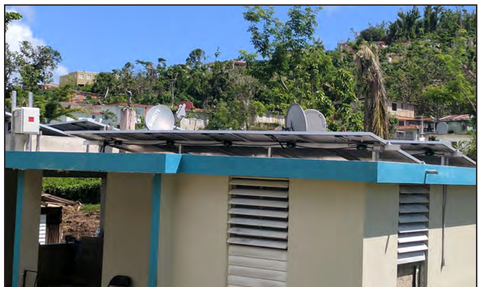
Figure 6-22: PV power system installed on a flat concrete slab roof in Naguabo with no visible damage.
