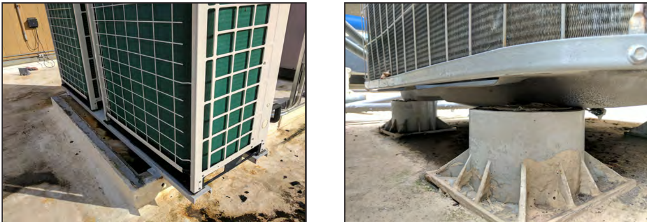
Figure 5-85: Rooftop equipment at Bayamón Municipal Building including, left, HVAC unit attached with screws to a curb; right, an AC condenser resting on plastic supports without anchoring. Rooftop equipment was not significantly displaced during Hurricanes Irma and Maria.
