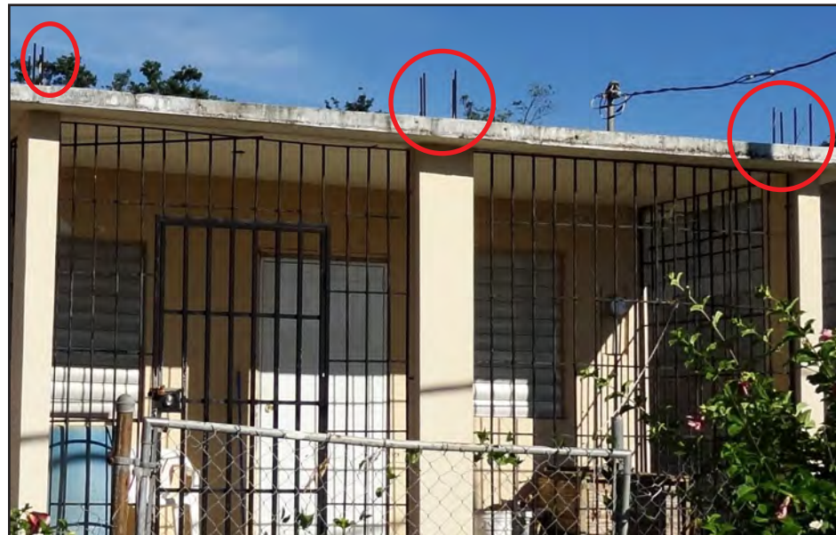
Figure 3-37: This home in Vieques had rebar exposed on the roof (red circles), indicating that the homeowner planned to add a second story sometime in the future.
