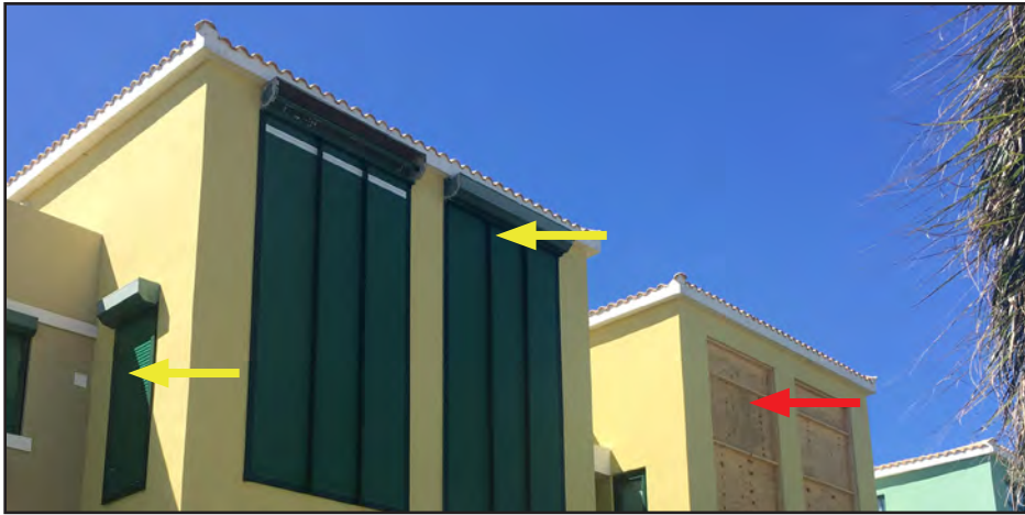
Figure 3-48: Residential windows, protected on the left (yellow arrow) and unprotected on the right, (red arrow) in Loíza. The unprotected windows were damaged and subsequently boarded up.
