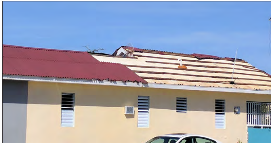
Figure 3-53: Residence with metal roof covering damage.
