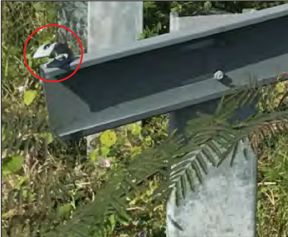
Figure 6-6: Reden solar array in Humacao: In this image, only the bent angle (red circle), remains after the steel lateral rail and bolted attachment were pried away in the hurricane.
