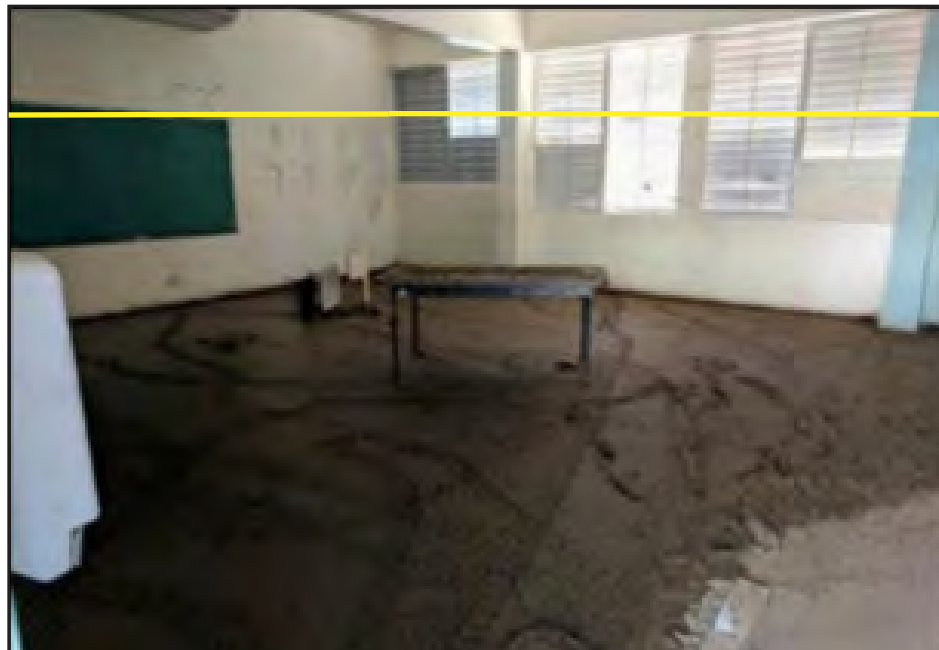
Figure 4-2: Mud remains in a classroom that was flooded (yellow line) at the Luis M. Santiago School, located in Zone AE.
