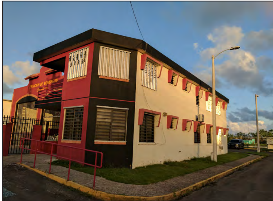
Figure 5-49: Metal shutters installed at the Luquillo Fire Station successfully protected the facility’s openings.
