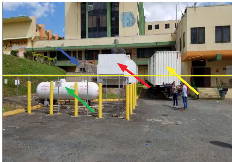
Figure 5-5: Dr. Ramon Ruiz Arnau University Hospital lower loading dock, which flooded from surface runoff, showing approximate high water level (red line), backup generator (red arrow), fuel tank (blue arrow), trailer mounted generator (yellow arrow), and propane tank (green arrow).
