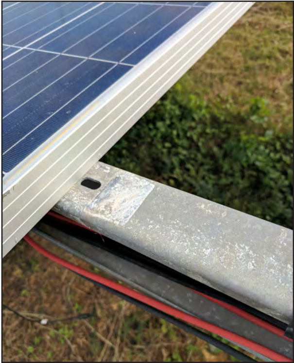
Figure 6-13: Oriana Solar Array 1: Steel lateral rail missing bolt and Hat-clip which held the adjacent PV panel.
