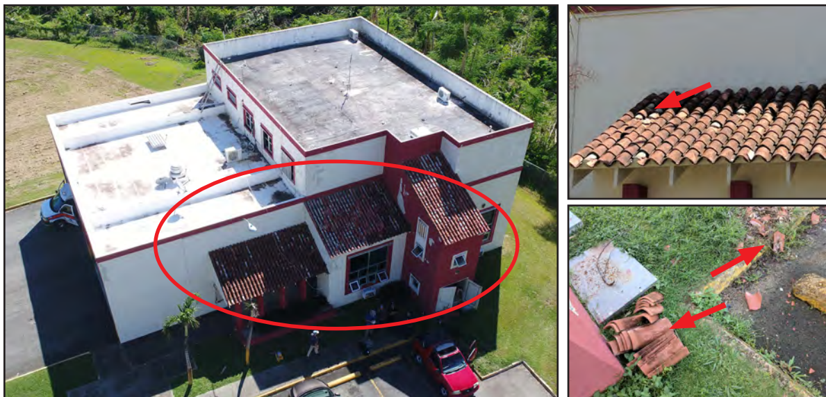
Figure 5-52: Damage to tile roof (red oval) covering at the Palmas del Mar Fire Station. Red arrows indicate broken tiles.
