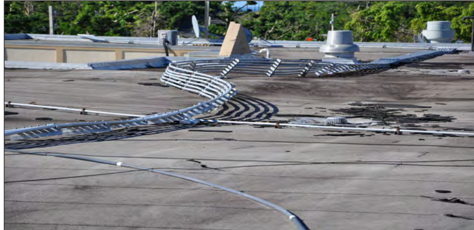
Figure 6-34: Failure of conduit connected to the roof used for the PV power system.
