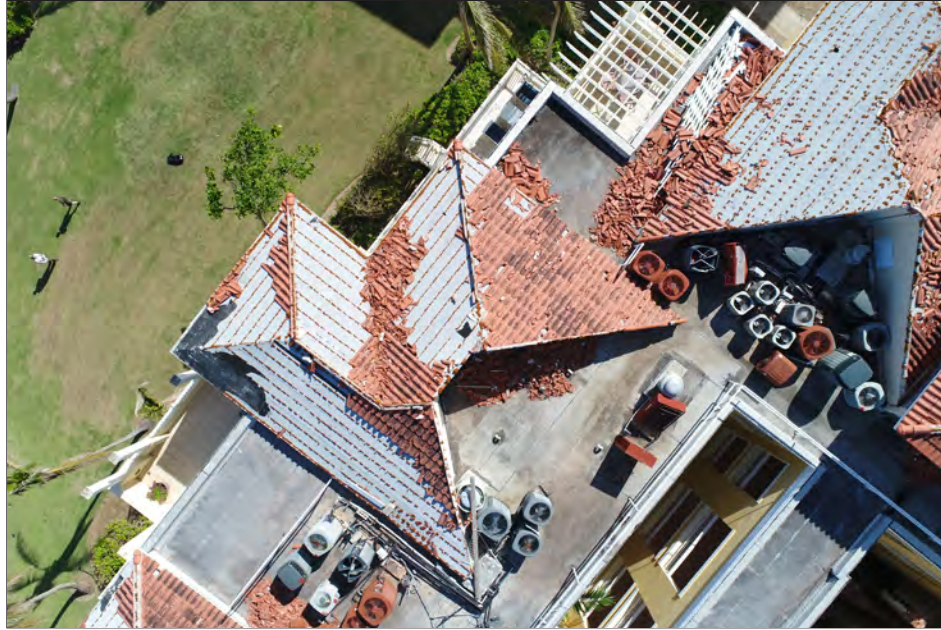
Figure 3-56: Tile roof performance with secondary protection from decking system. Tiles were removed, but the decking remained in place.
