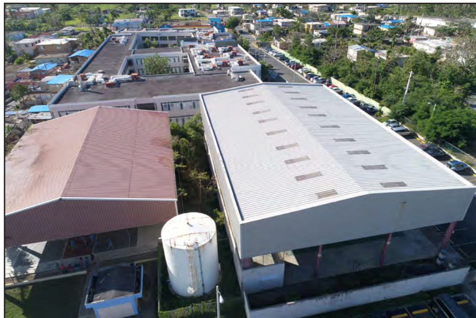
Figure 4-14: Two MBSs used as athletic facilities at Loíza Vocational High School that performed well and were not observed to have wind damage from Hurricane Maria.
