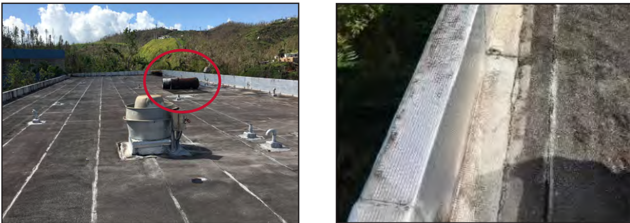
Figure 4-20: Modified bitumen roof covering at a school in Canóvanas. Left, water tanks (red circle) broke free of their attachments. Right, the roof covering is terminated and flashed on the backside of the parapet. This roof was approximately 2 years old and performed well during both Irma and Maria.
