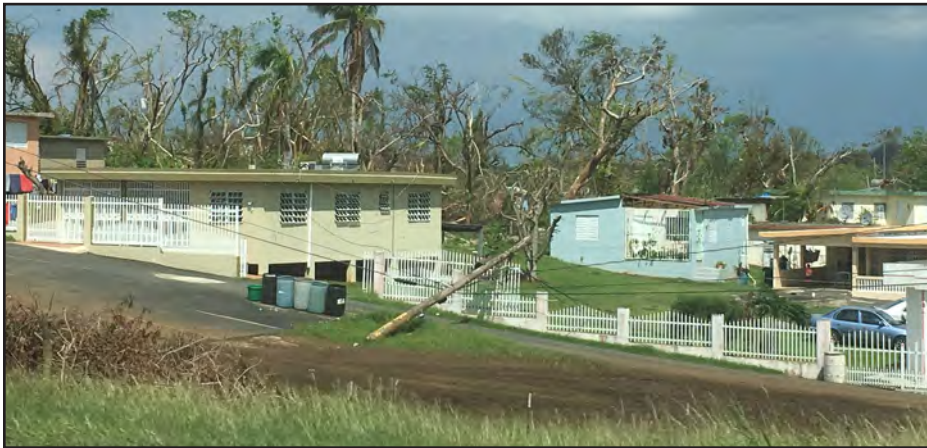
Figure 3-34: Comparison of two homes in Caguas: Left, the beige house had a reinforced concrete roof deck and experienced no structural damage; right, the blue CMU home lost most of its wood-framed roof and metal panel roof covering.
