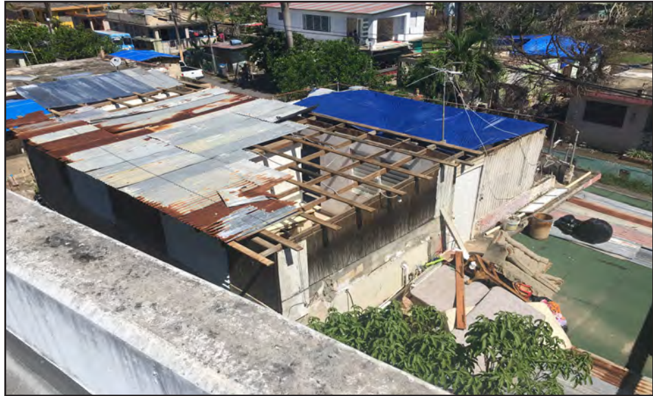
Figure 3-32: Informally constructed second story wood-framed addition in Loíza with partial loss of metal panel roof covering and wood-framed roof system.
