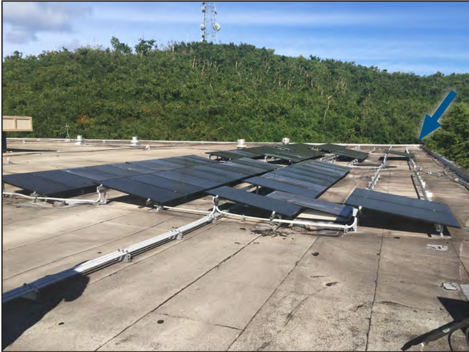
Figure 5-31: Rooftop solar array at east corner of hospital roof. The blue arrow indicates the direction of the strongest winds based on debris fields observed around the hospital.
