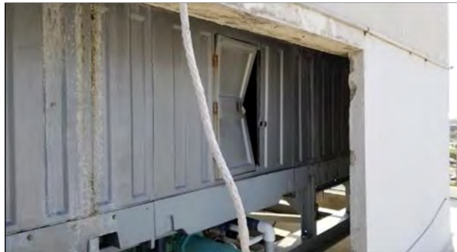
Figure 5-81: View of a service access door to the rooftop cooling towers atop the PRDOJ building. The door was driven into the cooling tower by debris impact (red arrow).
