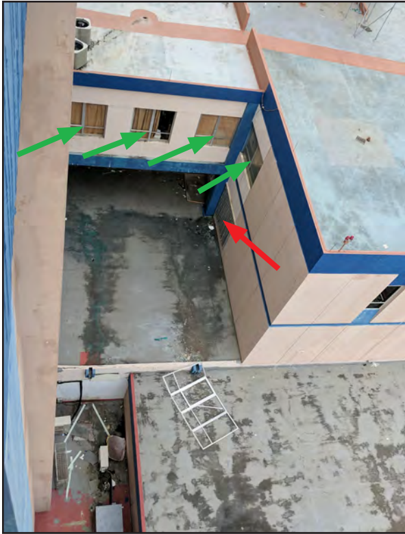
Figure 5-11: This view of Pavia Arcibo Hospital shows that some windows had glazing protection (red arrow) while others did not (green arrows).
