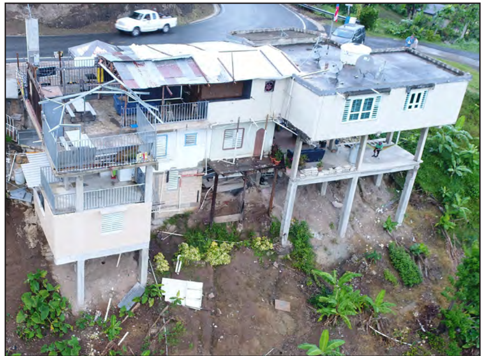
Figure 3-68: Hillside mixed-use building in Ciales with extensive lower-level additions at risk of landslide failure.
