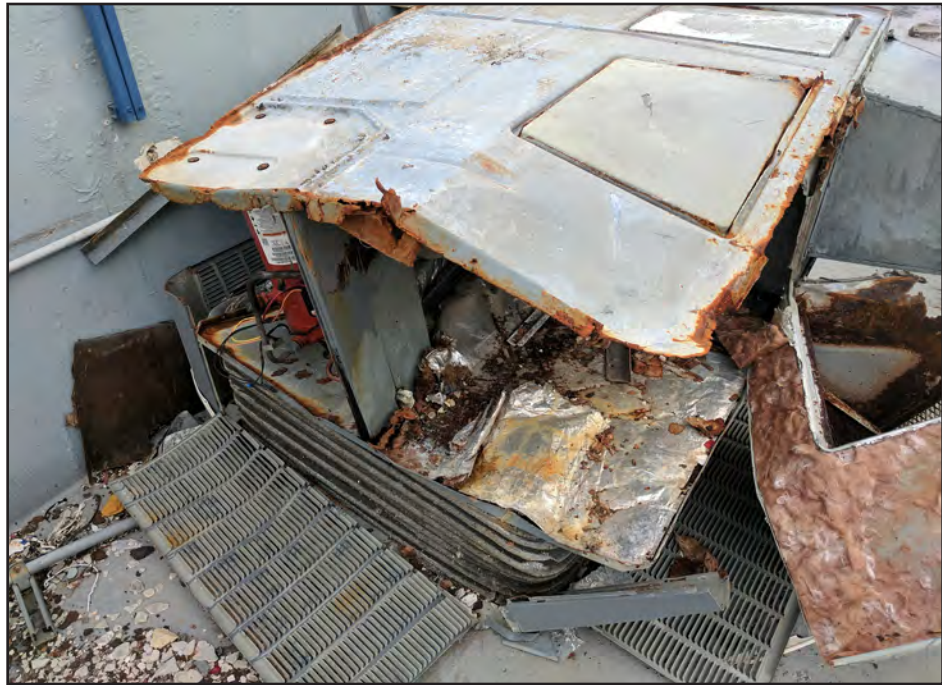
Figure 5-25: Damaged rooftop HVAC unit at Pavia Arcibo Hospital showing extensive corrosion. The unit is upside down and is missing side panels. The anchorage points on the bottom (now facing up) are rusted through and torn out.
