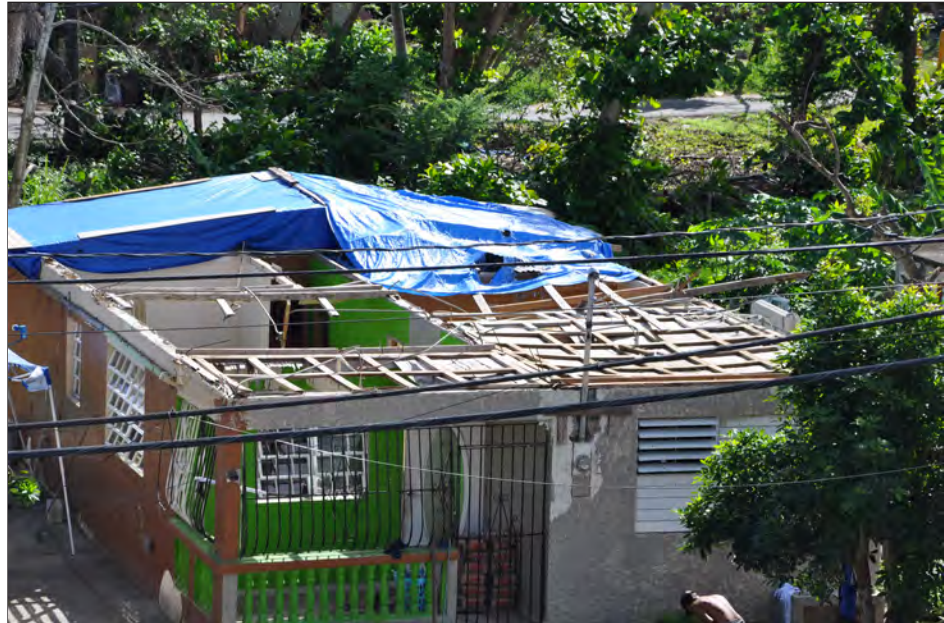
Figure 3-49: Residential building missing entire roof covering.
