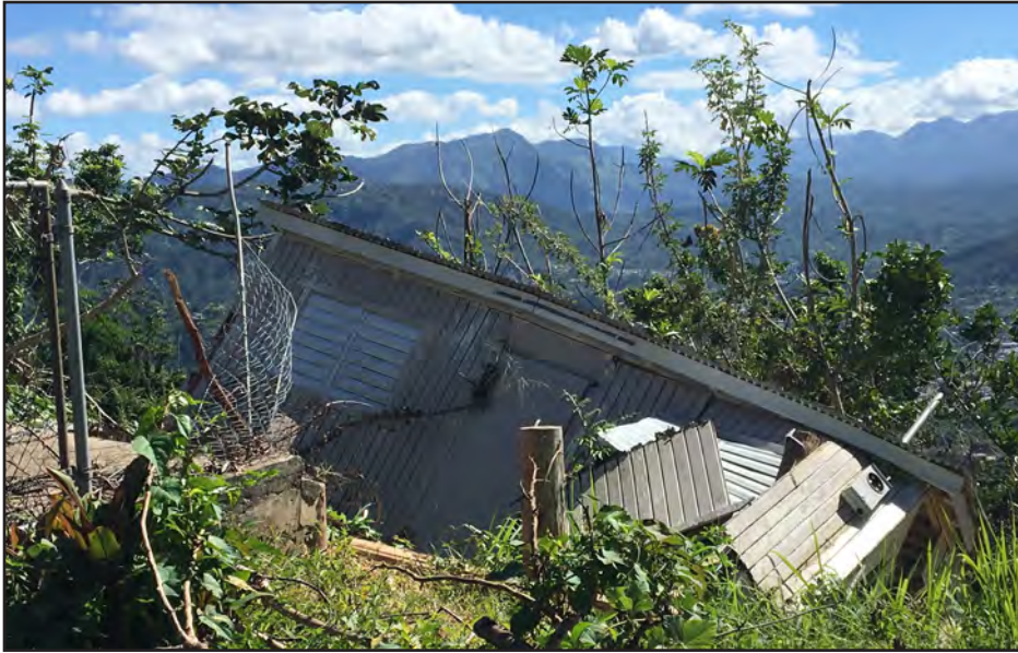
Figure 3-65: Hillside residence in Cerro Gordo, Utuado that failed due to poor siting on unstable slope and poor connection of wood foundation to building.
