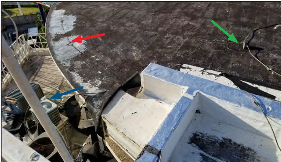
Figure 5-78: The lightning protection air terminals (green arrow) tore free from their anchorages (red arrow) atop the PRDOJ building. Rooftop AC units were also displaced (blue arrow).
