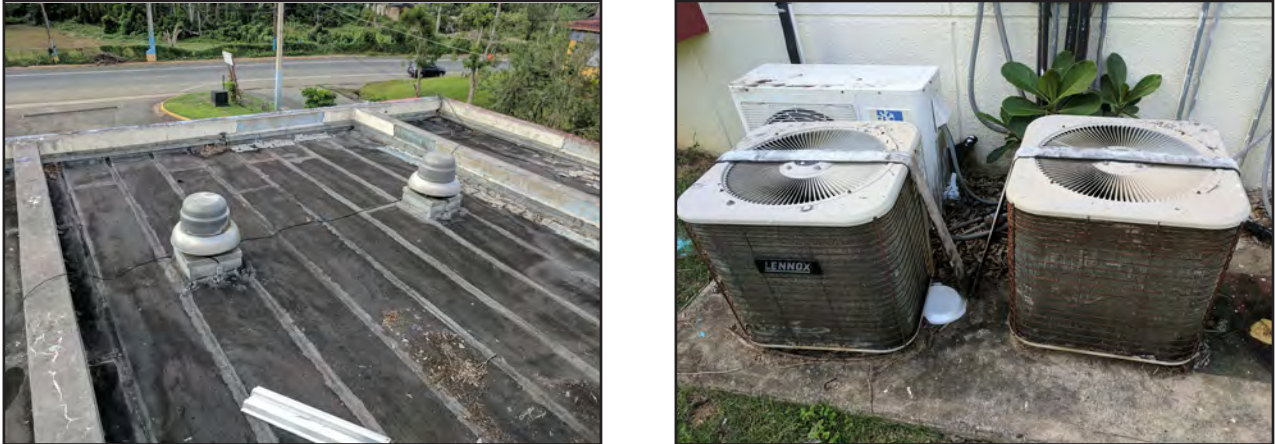
Figure 5-55: Florida Fire Station, with, left, minor roof damage, right, strapped AC condensers.
