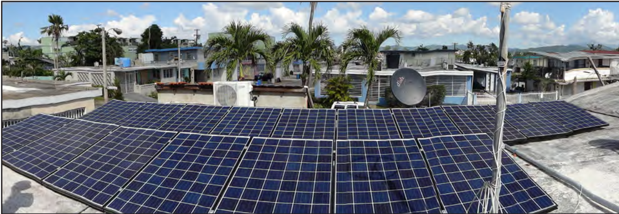
Figure 6-23: PV power system installed on a flat concrete slab roof in Caguas with no visible damage.
