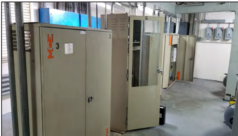
Figure 5-39: Elevator controls that were inundated with wind-driven rain and failed during the hurricane at Dr. Ramon Ruiz Arnau University Hospital.
