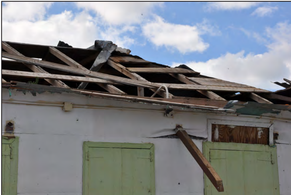
Figure 3-51: House with metal roof and nailers pulled from its roof structure with no structural decking.
