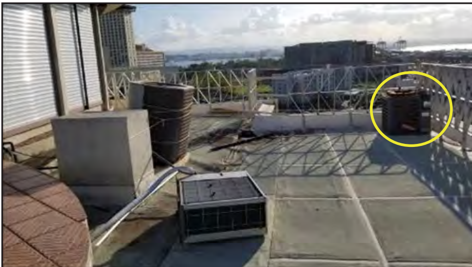
Figure 5-79: HVAC equipment was blown off equipment pads at the roof level of the PRDOJ building. One HVAC condenser has been blown to the edge of the building (yellow circle).
