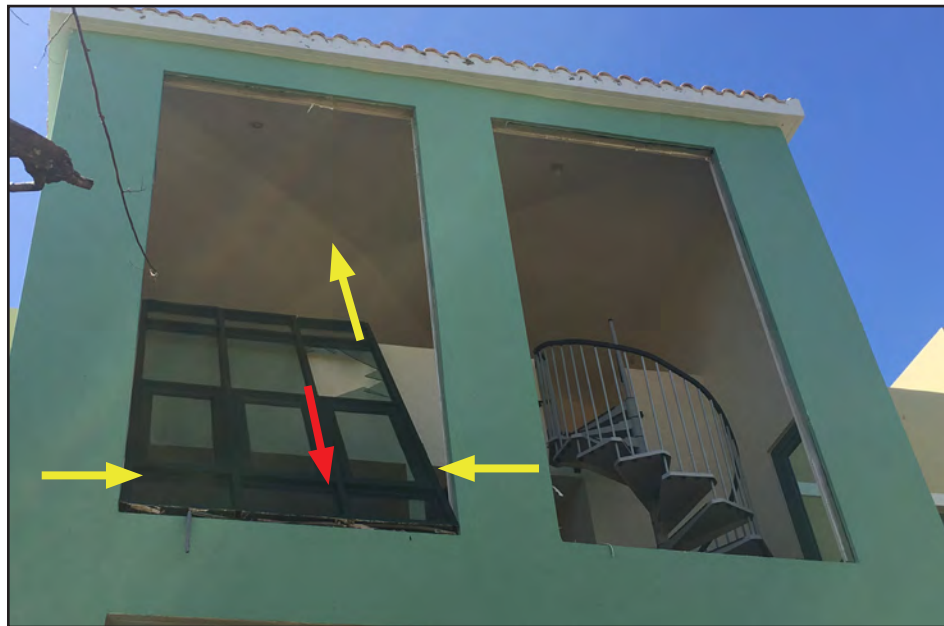
Figure 3-41: Low-rise residential building with large glazed windows blown in (yellow arrows) and windows broken (red arrow).
