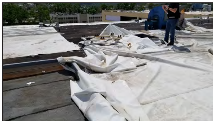
Figure 5-19: The roof membrane over the central section of Dr. Ramon Ruiz Arnau University Hospital peeled off over most of the roof, allowing water intrusion into the floors below.
