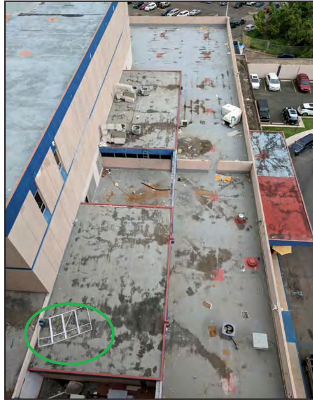
Figure 5-12: At Pavia Arcibo Hospital, a window frame was pulled out of the building (green circle). The frame was inadequately anchored to the wall opening.
