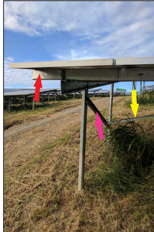
Figure 6-11: Oriana Solar Array 1: The brace connecting each row of posts (pink arrows) provides additional strength to the posts and helps limit the overall sway or movement of the PV array perpendicular to the lateral rails (red arrow). The yellow arrow in the image points to a brace which connects posts parallel to the lateral rails. This brace will assist the system in a similar manner in the opposite direction.
