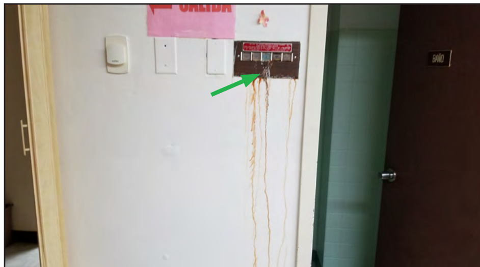
Figure 5-13: Rain water from the fourth floor of Dr. Ramon Ruiz Arnau University Hospital, Bayamón, migrated to the lower floor through floor penetrations and inundated numerous systems including electrical conduits and communications boxes (green arrow).
