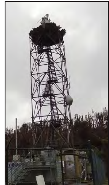
Figure 6-43: Failure of radar bubble on communication tower in Cayey. The tower itself appeared undamaged.
