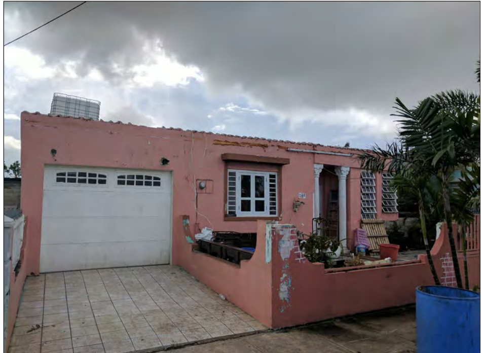
Figure 3-74: This NSHP house in Campanilla Toa Baja suffered damage to aesthetic components including clay tile roof coverings and decorative eaves blown off by wind.
