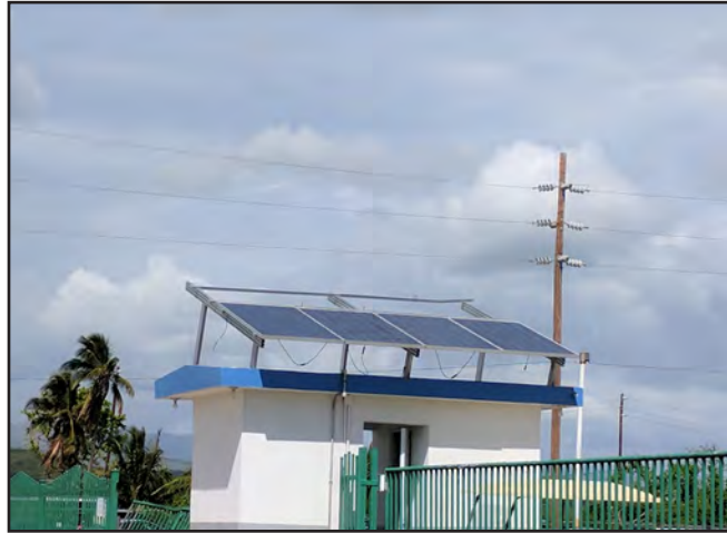
Figure 6-39: PV power system at Zimmer Biomet in Mercedita, Ponce, which lost four of its eight panels.
