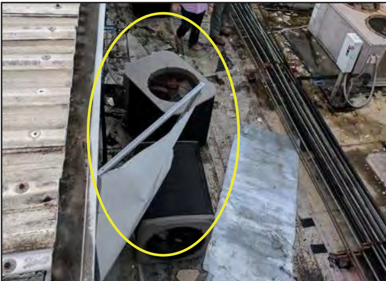
Figure 5-83: View of rooftop mechanical equipment displaced (yellow circle) and damaged by the hurricane winds.
