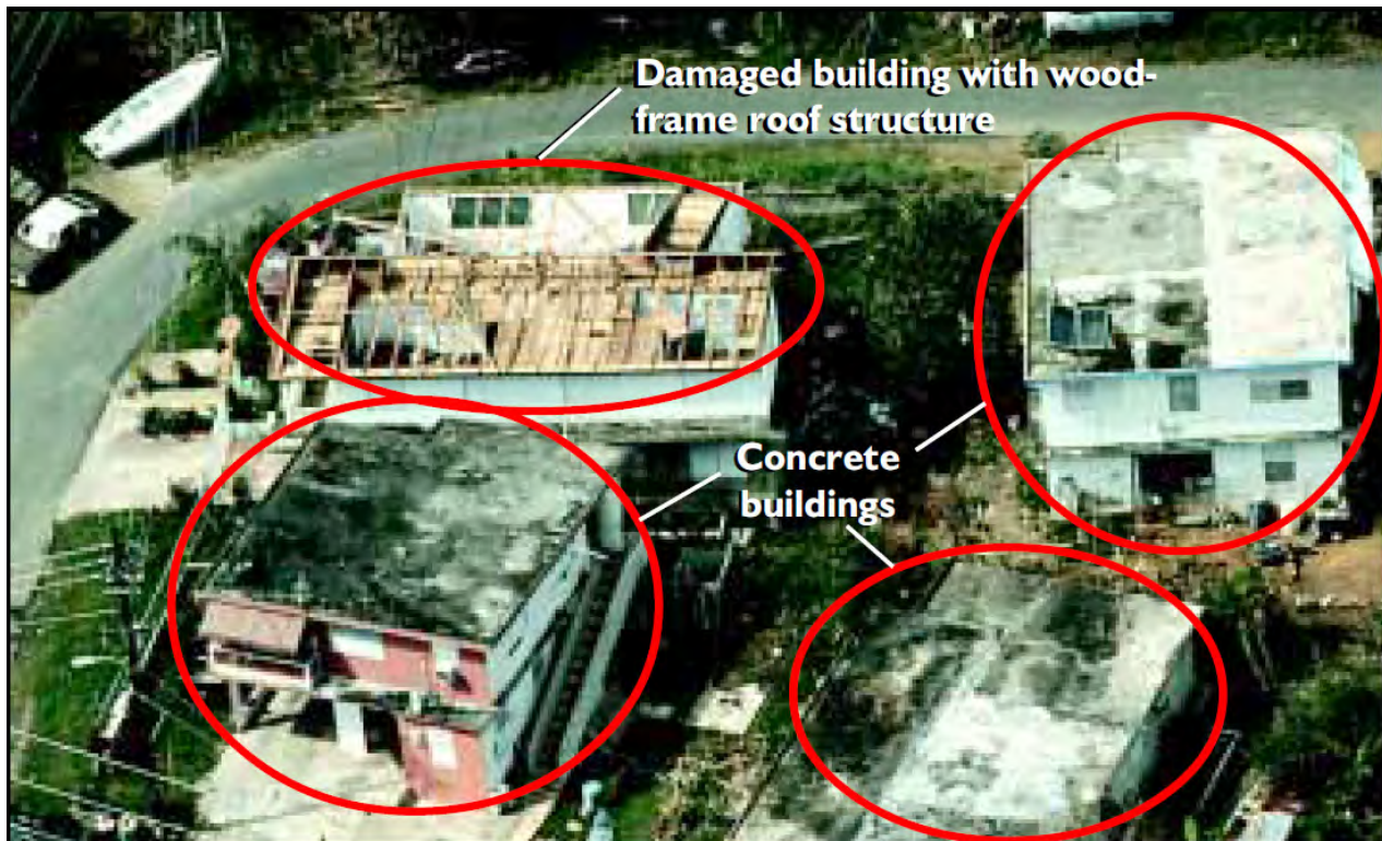
Figure 1-13: Examples of observed damage by the BPAT after Hurricane Georges in 1998. Source: (FEMA, 1999a).
