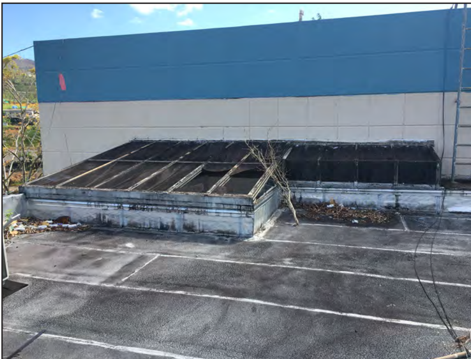
Figure 4-19: Broken skylight glazing at a high school in Canóvanas.
