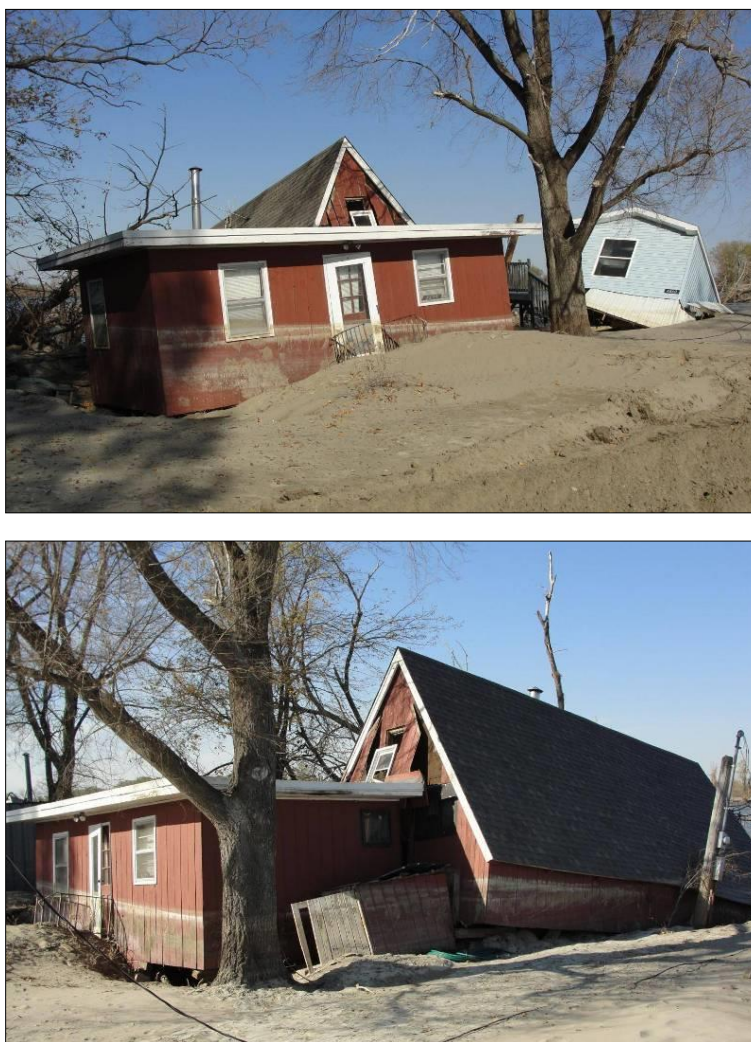
Figure 9-1: Two views of the same structure showing a high water mark, structure displacement, and some of the damage
