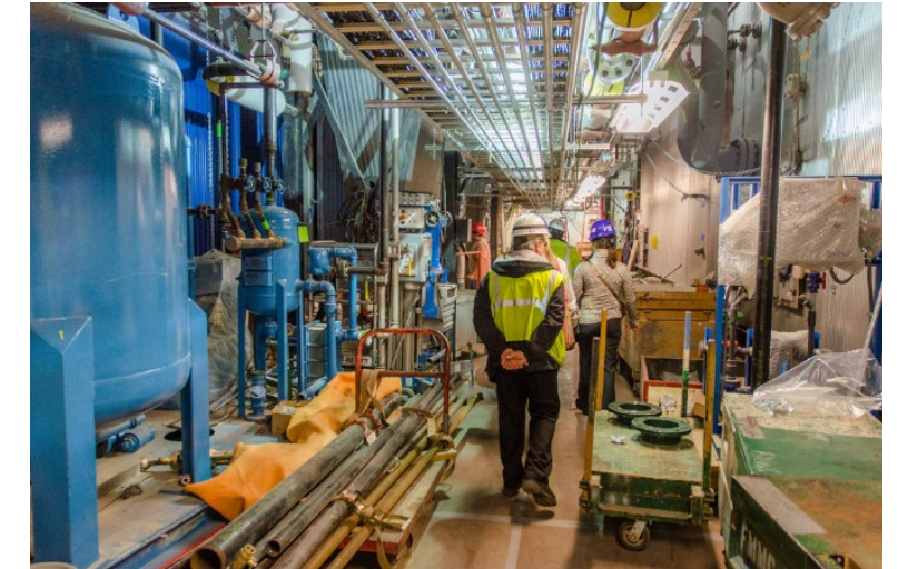
NYU Langone Medical Center Generators Source: FEMA
