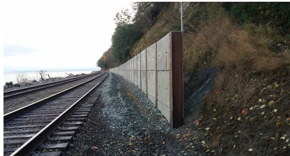
Landslide Mitigation retention wall: The finished metal and concrete landslide retention wall helps keep debris from covering the tracks.
