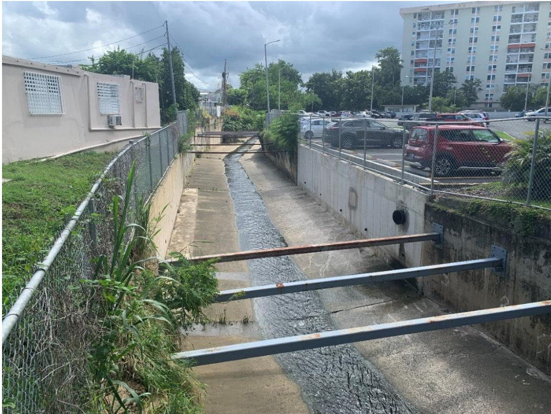
Figure 1-3: Trapezoidal channel concrete walls failing along the Quebrada Buena Vista Stream, between the Jardines Metropolitanos residential building complex and the Ramón Nevárez community in San Juan. (2023).
