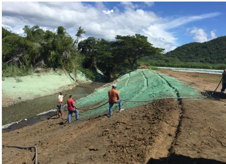
Figure 2-1: Hydroseeding performed by Protectores de Cuencas to help restore the banks of the Río Loco in Yauco (Photo credit: PDC)
