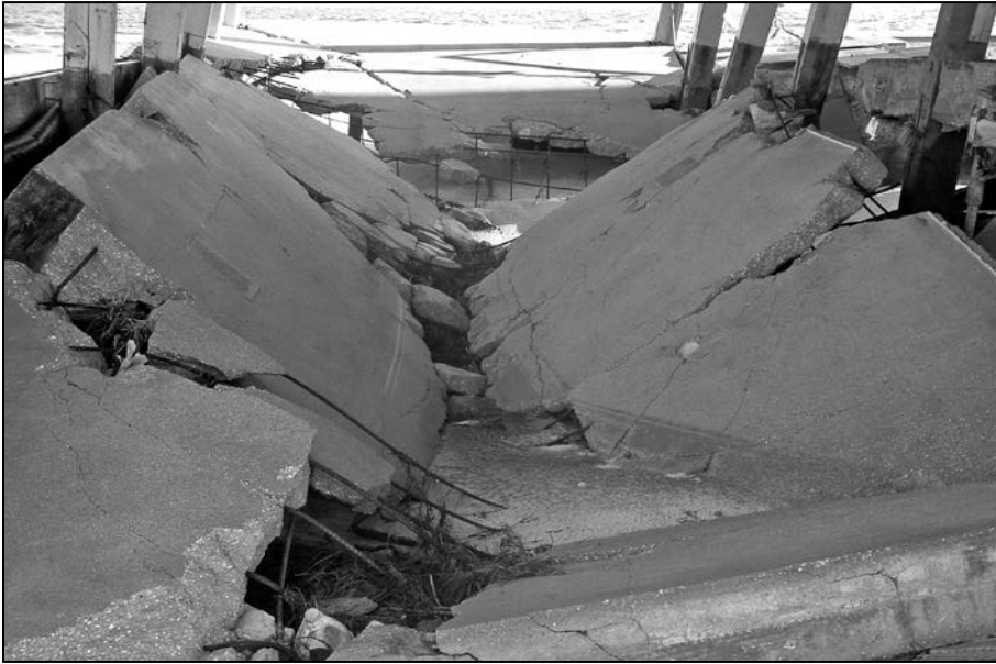
Figure 20: Damage to building foundation caused in part by failure of the reinforced slab undermined by erosion
