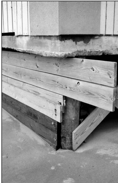
Figure 25: Shore-parallel timbers attached to a pile foundation that were intended to act as a bulkhead but constituted an obstruction and are not permitted
