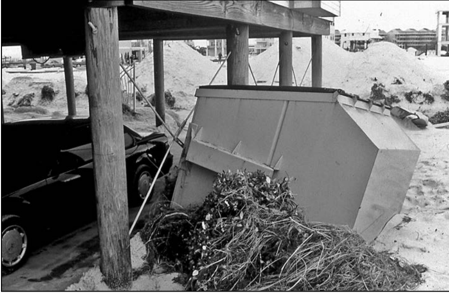
Figure 14: Floating debris trapped by metal rod cross bracing
