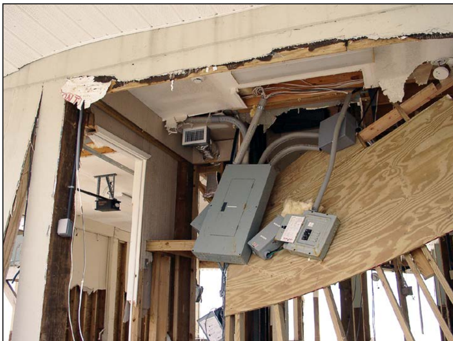
Figure 13: Utilities mounted on wall, which prevented the wall from breaking away cleanly
