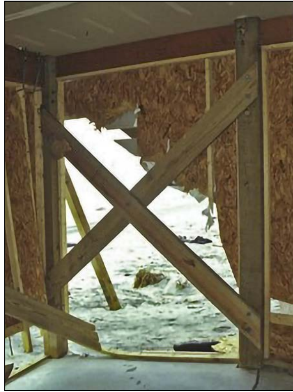
Figure 16: Cross bracing that interfered with the failure of a breakaway wall
