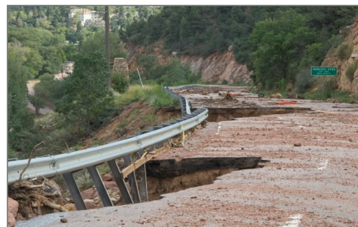
A road is severely damaged by flooding in Manitou Spring, Colorado, 2013.
