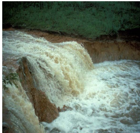
Figure 2.3.11. Headcut erosion could lead to an accidental release from the impoundment. (Source: NRCS, 2017)
