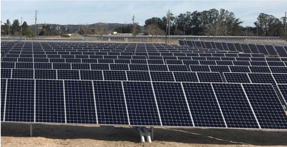
Figure 4.3.14. A solar array on Vandenberg Air Force Base helps power facilities on the base. (Source: Defense Logistics Agency, photo by Airman First Class Clayton Wear, No Date)
