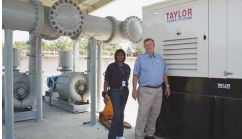
Figure 4.1.3. Installing an emergency backup generator can provide power to help a water treatment plant continue to operate during a flood. (Source: U.S. Environmental Protection Agency [EPA], 2014)
