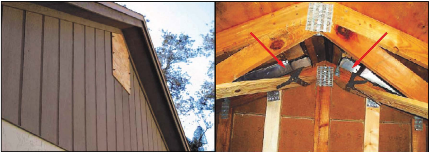
Figure 3.3.1.11. Protecting gable end vents using shutters (left) and sealing gable rake vents using metal plugs as indicated by red arrows (right).
