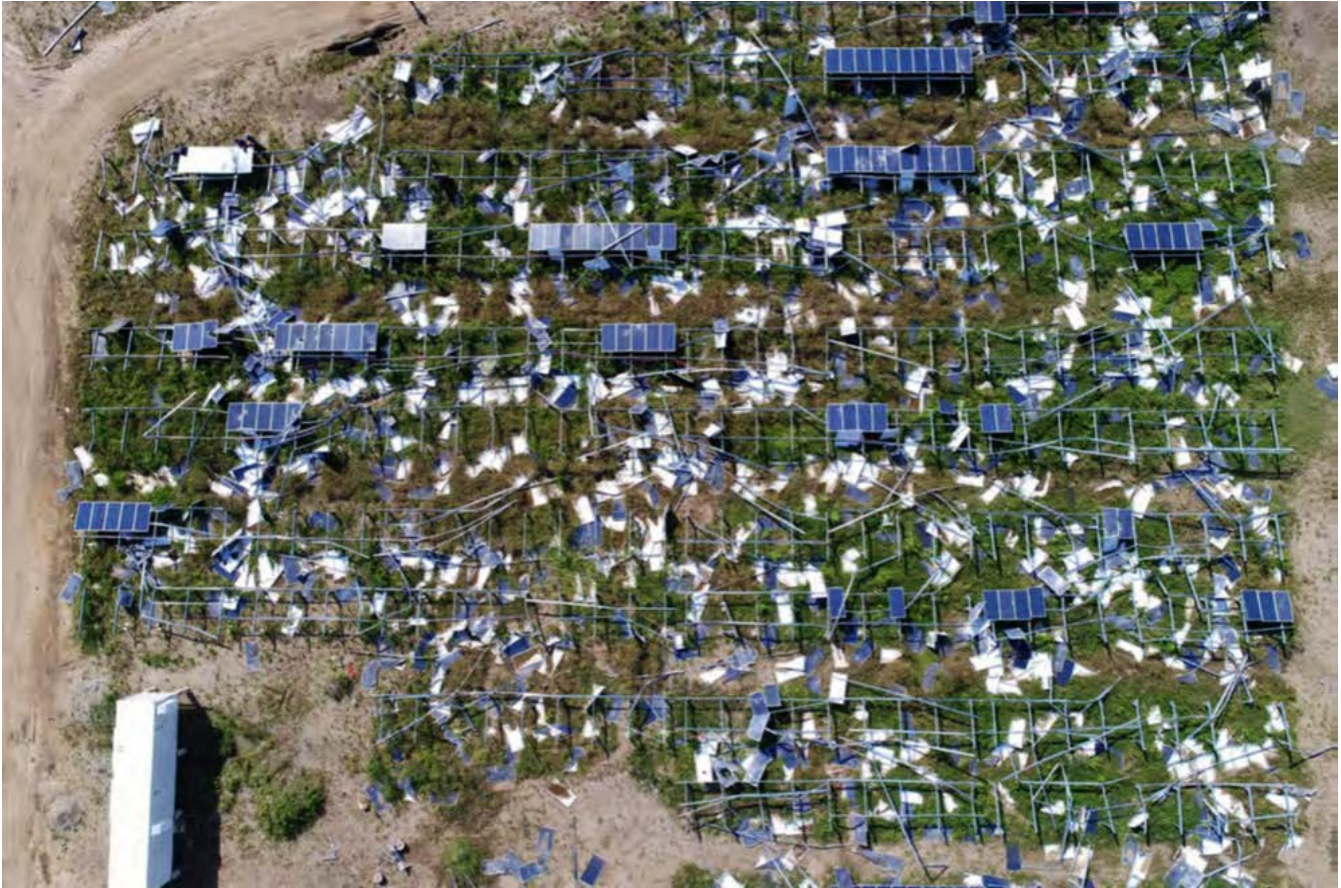
Figure 4.3.12. Hurricane Maria severely damaged a solar array in Puerto Rico in 2017.
