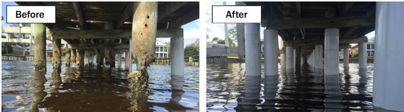
Figure 5.5.2. Fit aging piles with jacket encasements to strengthen and protect them (Source: Shoreline Plastics, No Date).
