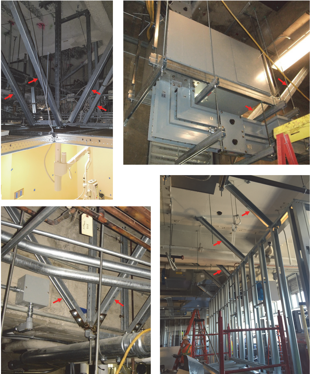
Figure 9-2 Examples of nonstructural bracing. Top left: Ceiling-mounted medical device. Top right: Above-ceiling air handling unit (from FEMA E-74). Bottom left: Conduit (from FEMA E-74). Bottom right: Partial-height partition wall. Red arrows point to braces.
