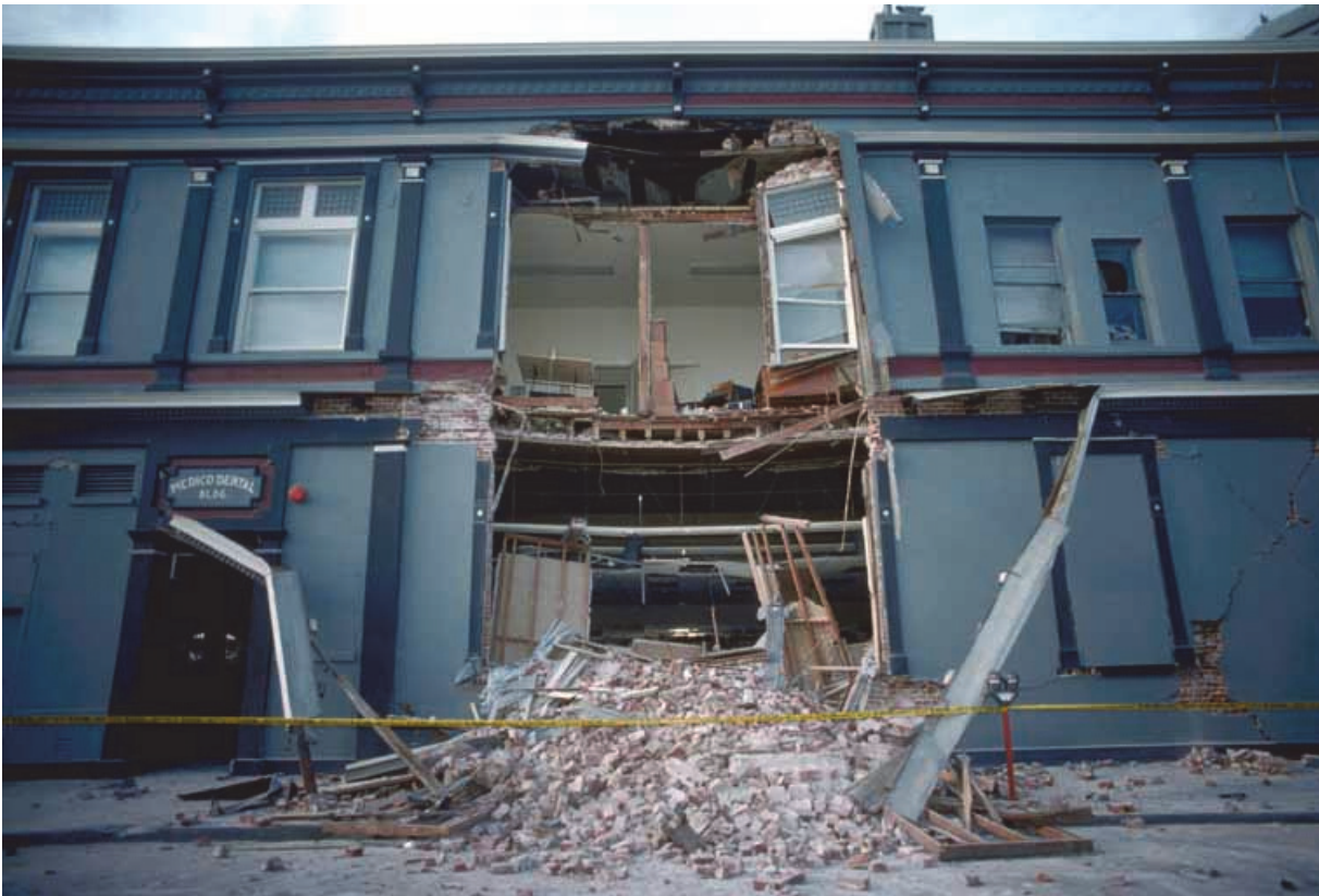
Figure 4-14 Failure of an unreinforced masonry wall in the 1989 Loma Prieta Earthquake (from USGS).
