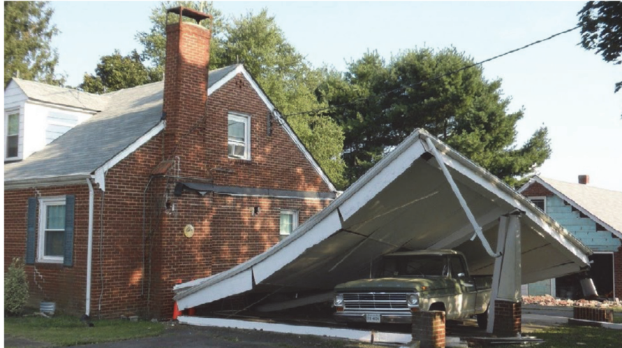
Figure 4-5 This carport, originally supported by but not firmly attached to the adjacent house, became detached from the house during ground shaking (from FEMA P-530).
