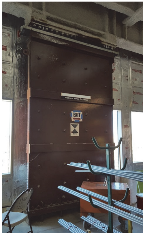
Figure 5-11 Wall damper visible during construction of a hospital.
