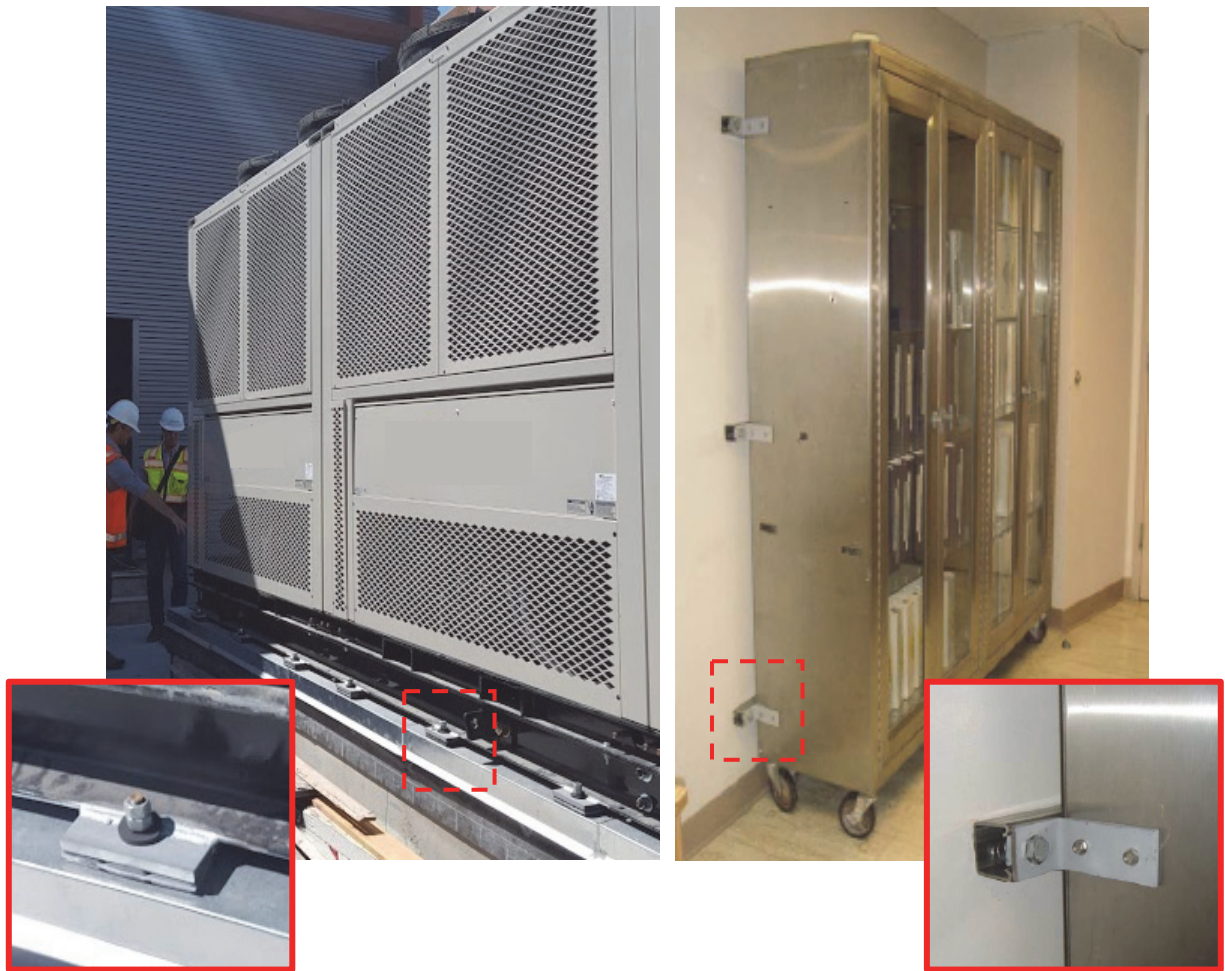
Figure 9-1 Examples of nonstructural anchorage. Left: Rooftop air handler anchored to a housekeeping pad. Right: Shelving unit mounted to a wall (from FEMA E-74).
