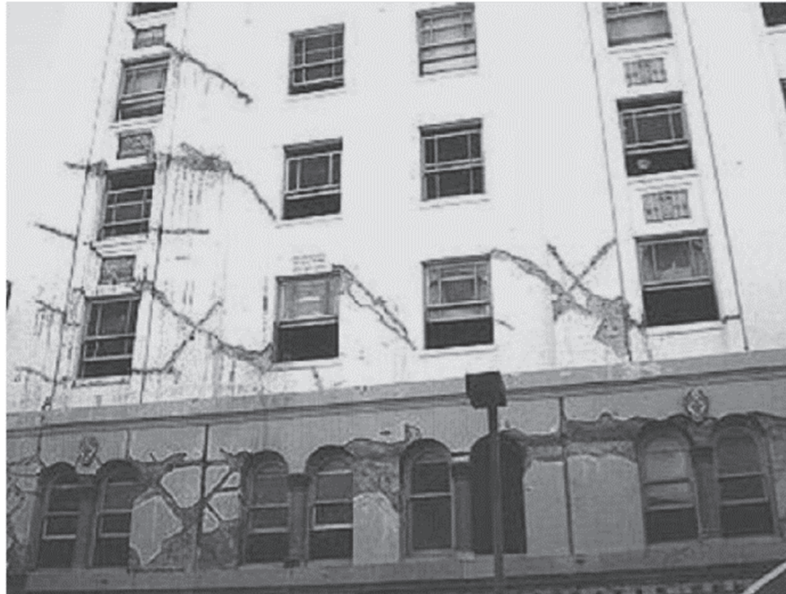
Figure 5-6 Diagonal cracking in a reinforced concrete building damaged by the 1989 Loma Prieta Earthquake (from FEMA P-154).
