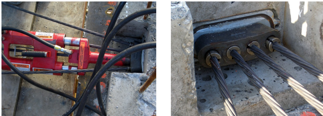
Figure 8.38 – Mono-Strand Stressing of a 4 Strand Tendon (left). Anchorage After Stressing 2 nd Strand (right).
