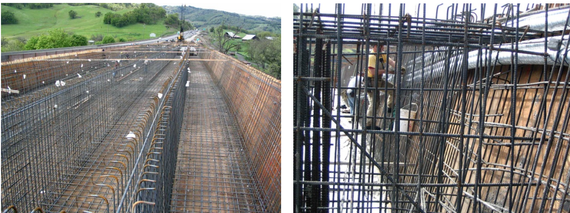
Figure 1.21 – Web and Bottom Slab Reinforcing (left), Tying Post-tensioning Ducts in Webs (right)
