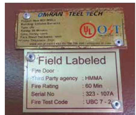
SIGAR inspectors at the U.S.-funded Ministry of Interior compound in Kabul found that contractors had installed hundreds of non-certified, non-factory-labelled fire doors, some including fake logos of Underwriters Laboratories. (SIGAR photo)
