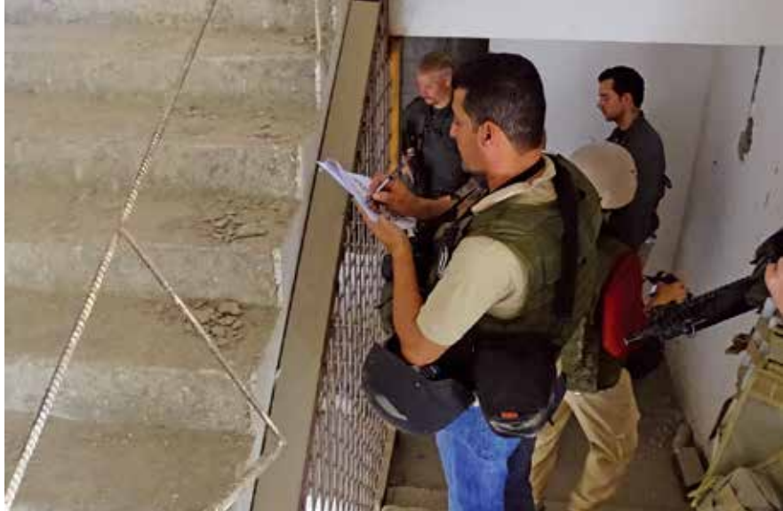
SIGAR engineers inspect unfinished construction at a Kabul hotel project that was backed by a U.S.-guaranteed loan. (SIGAR photo)
