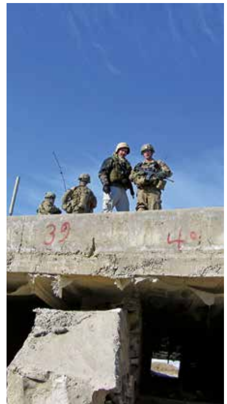
A SIGAR investigator traveling with U.S. military personnel confirmed that anti-terrorist gratings had been falsely reported as installed at this highway culvert. A court proceeding related to the fraud was conducted in July 2017. (SIGAR photo)
