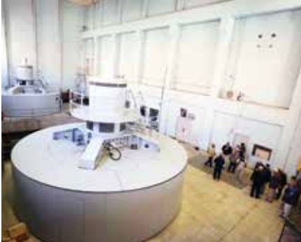
U.S. officials view the dynamo room at the Kajaki Dam. (U.S. State Department photo by Musadeq Sadeq)
